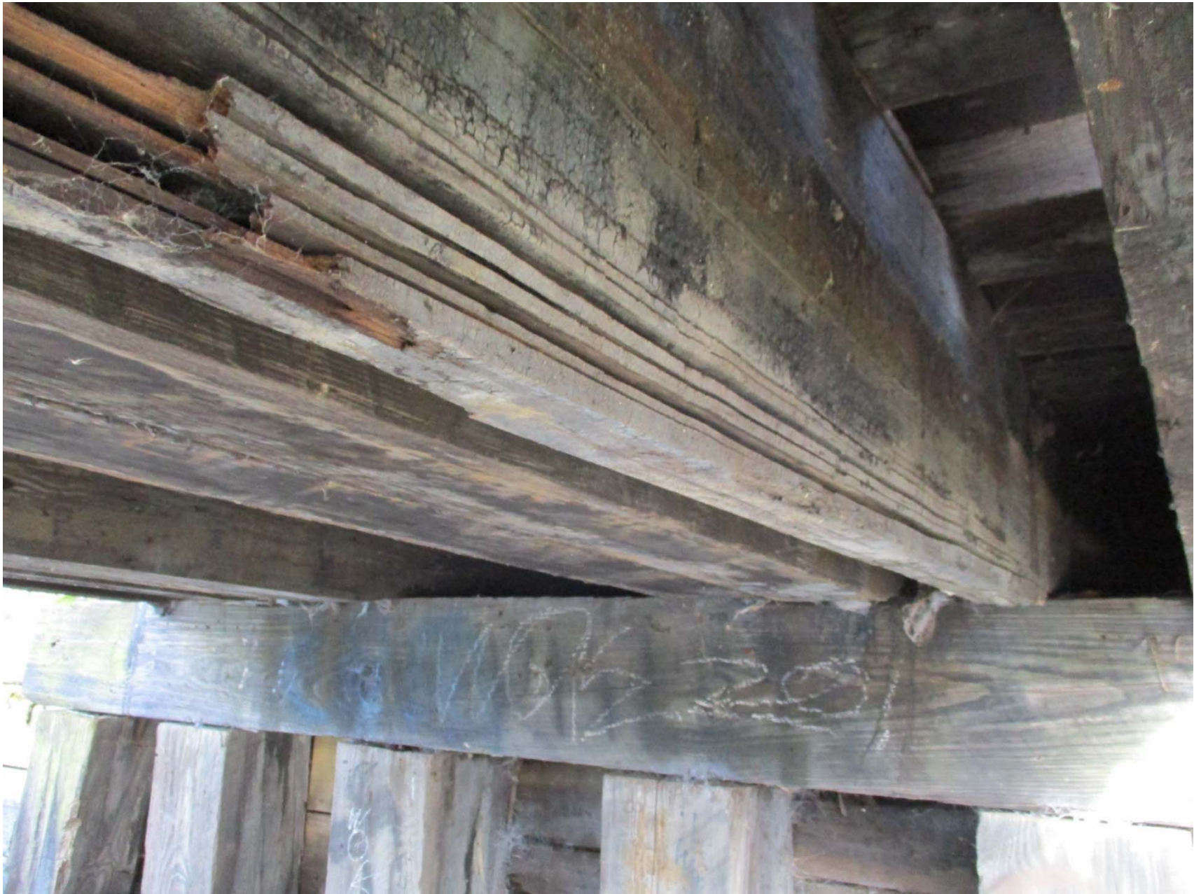
Splitting along bottom of beam 2E at north abutment
