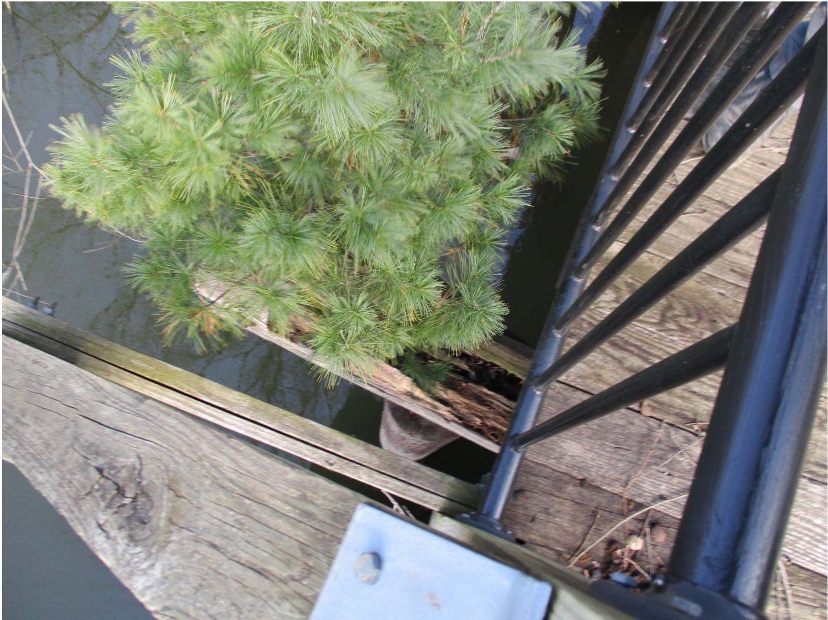
Pier 9S west end rotted with 4ft white pine
