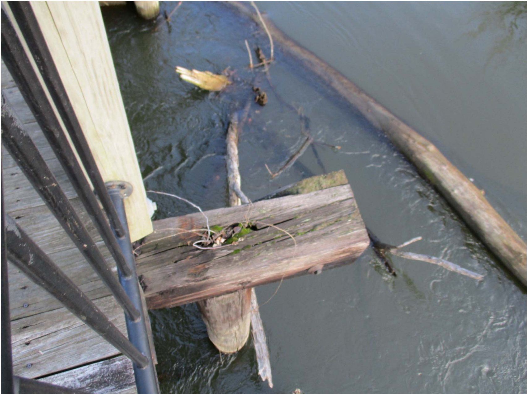
Pier 6S east end with internal rot
