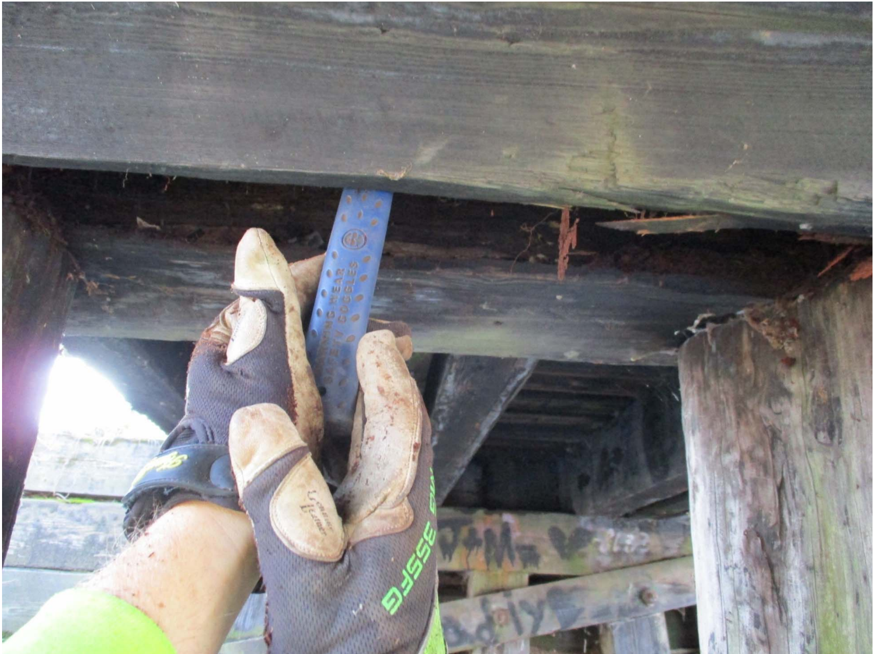
Pier 1S internal rot in east half
