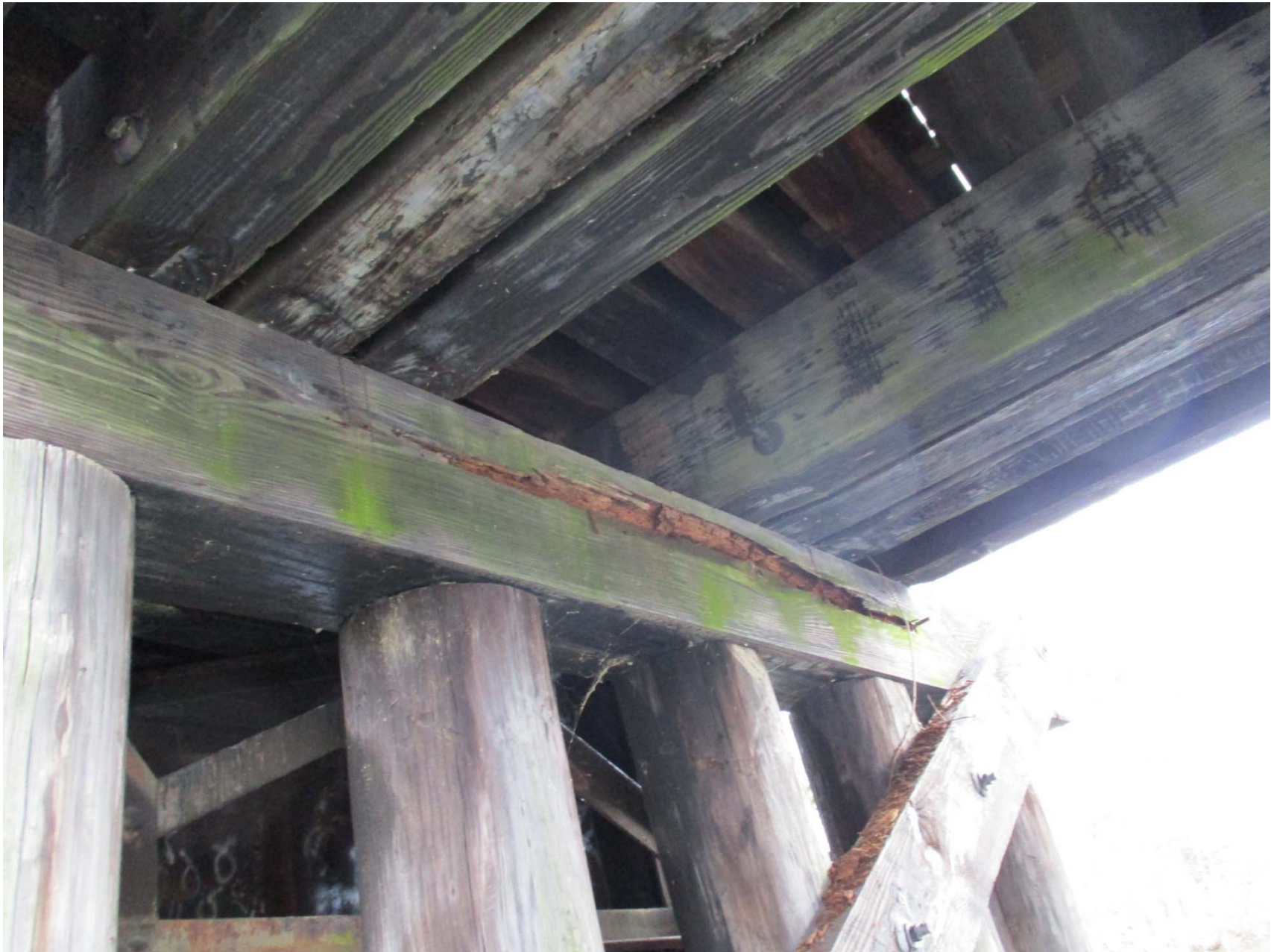
Pier 7S rot along the side 3" deep
