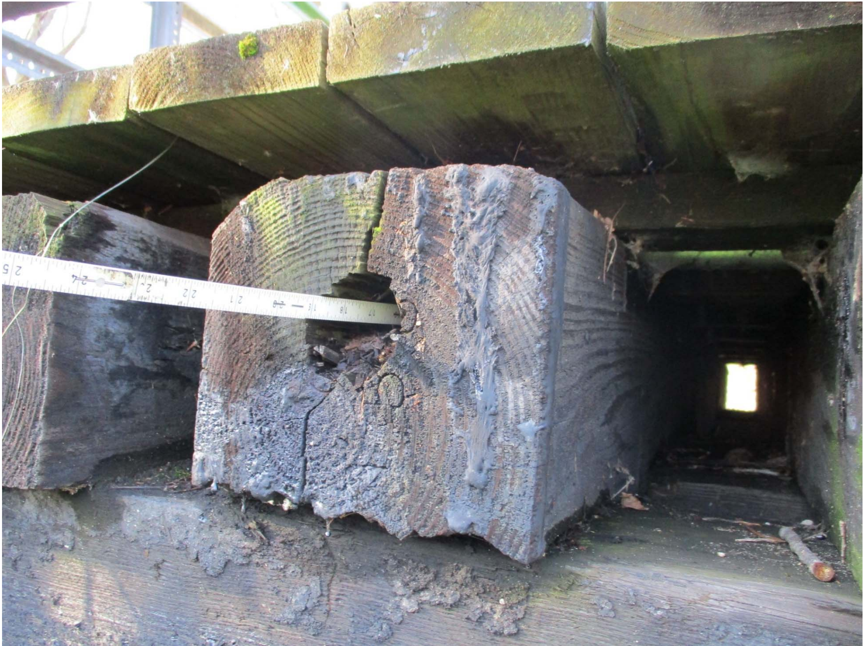
Tie end rot at south abutment
