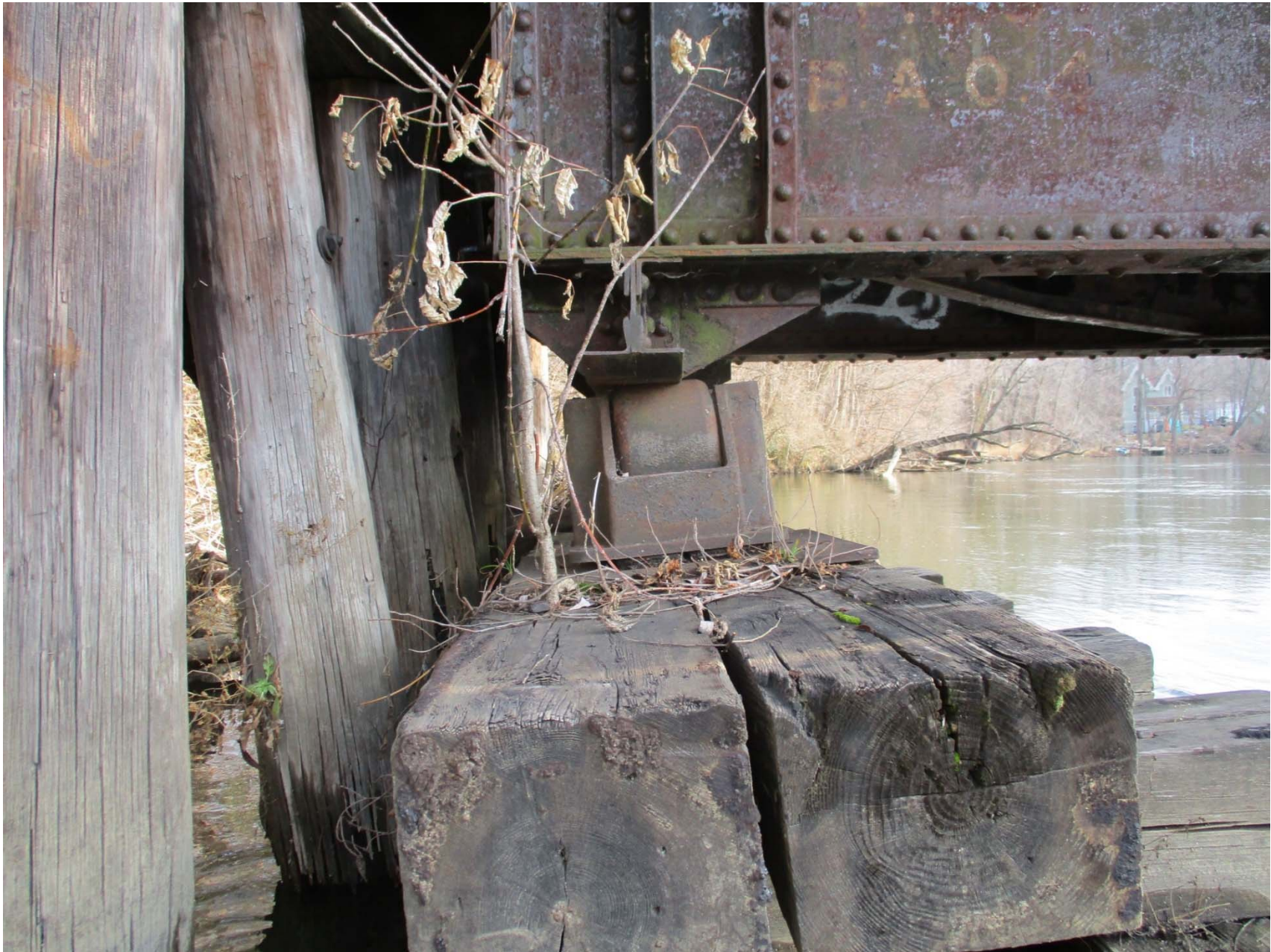
West bearing at pier 9S cribbing rotated
