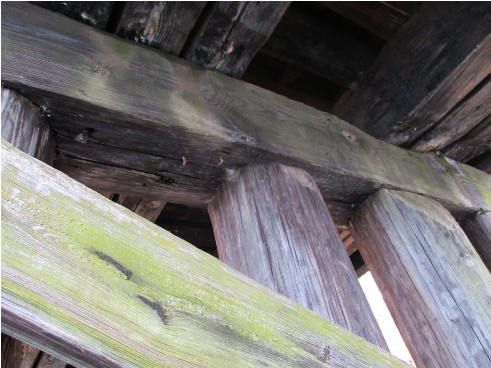
Pier 10S bottom of cap split
