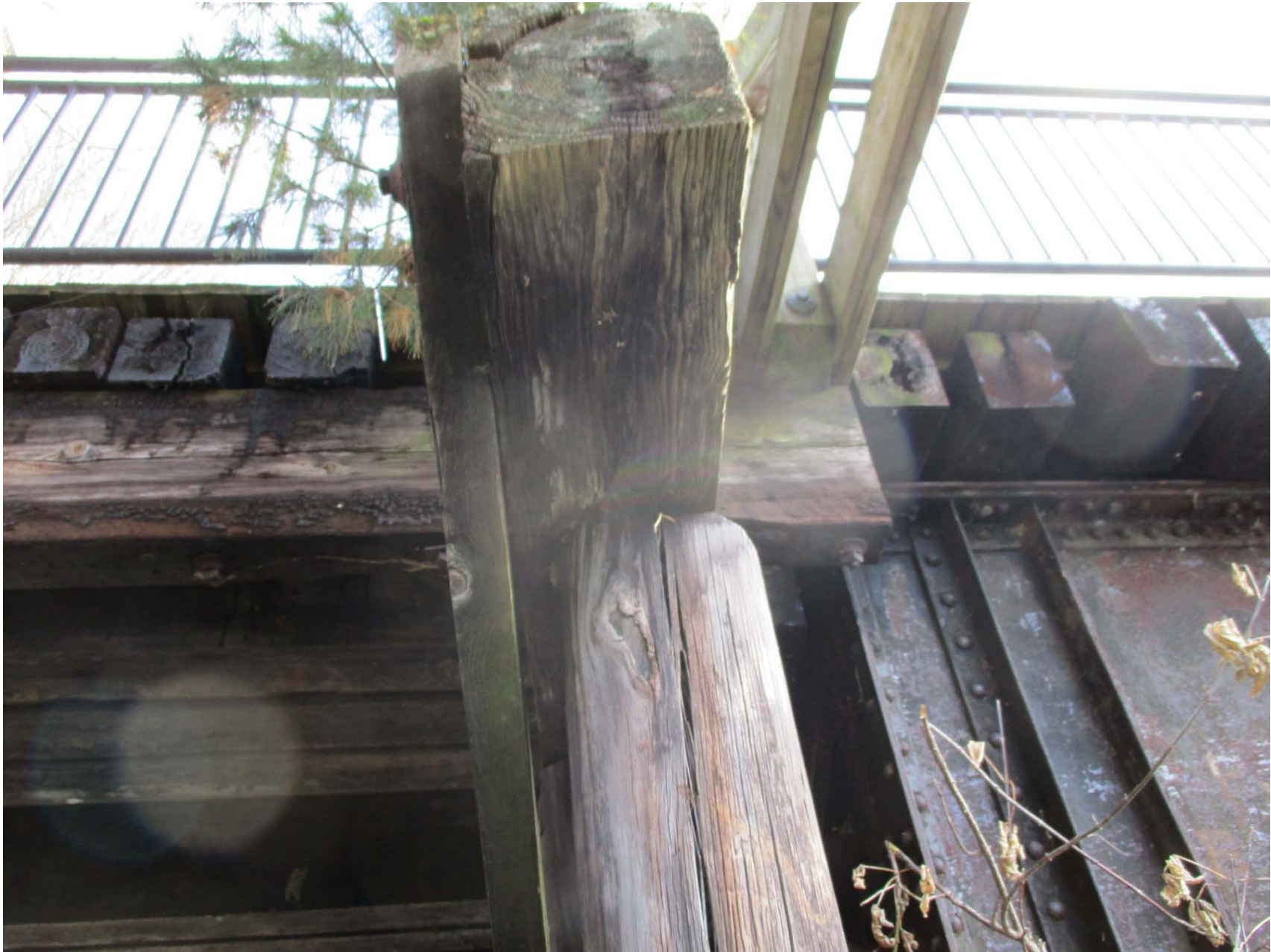
Pier 9S west end of cap offset
