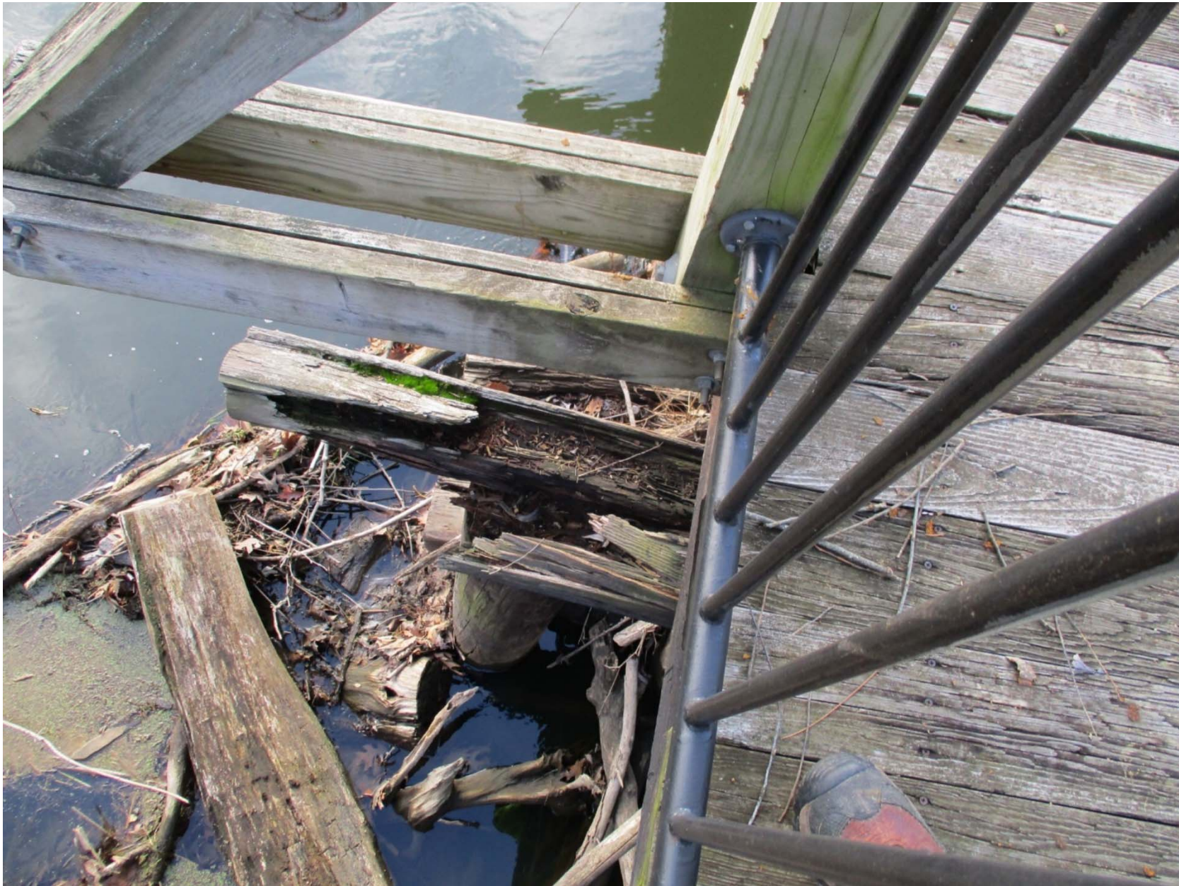
Pier 9S east end nearly rotted through
