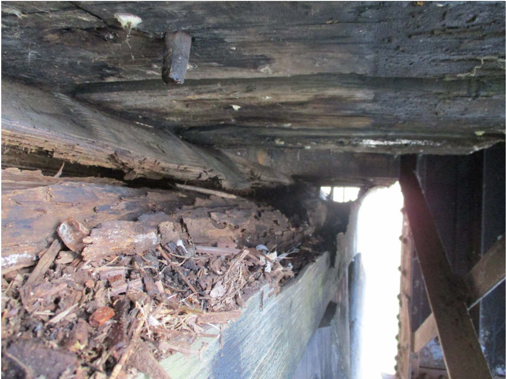
Top of pier 9S rotted full width for length of the cap, no beam support remains
