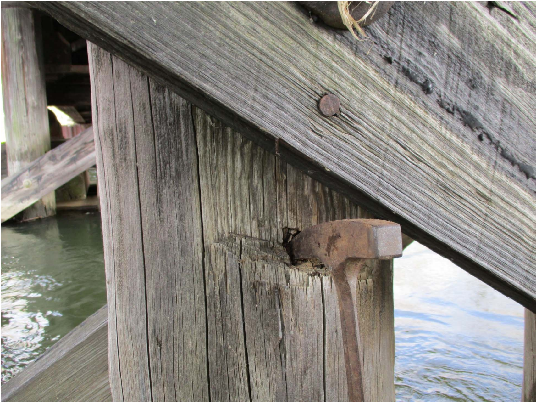
Pier 6S pile 3W has some internal rot
