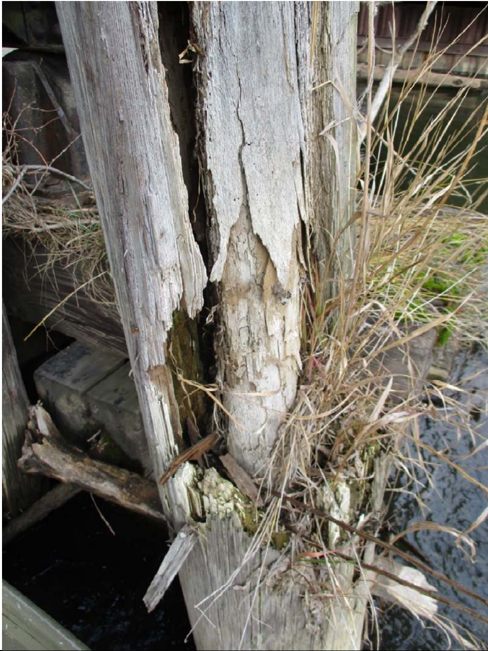
Pier 7S pile 1E nearly rotted through
