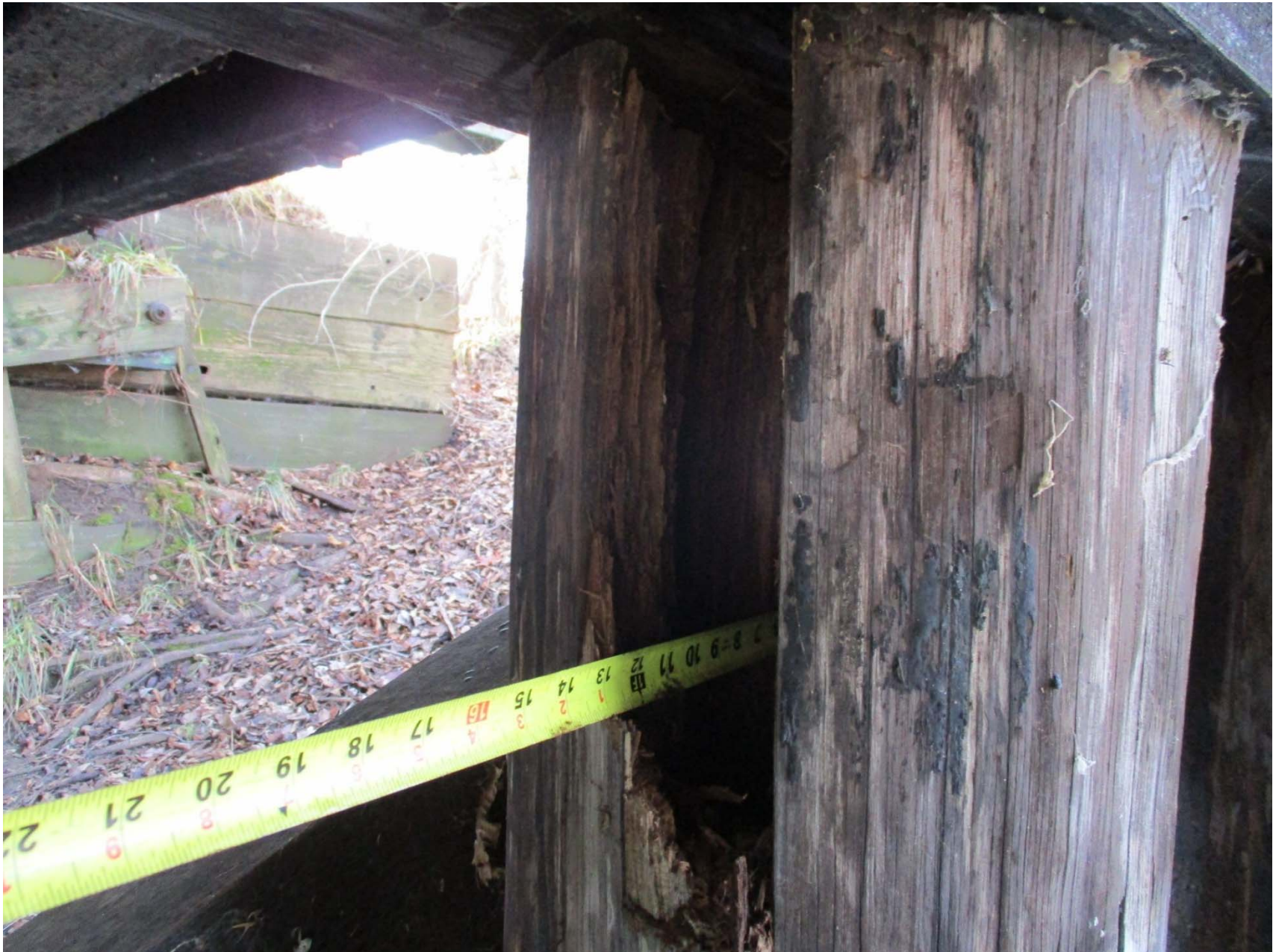
Internal rot in pile 2W exposed, only outer shell remains
