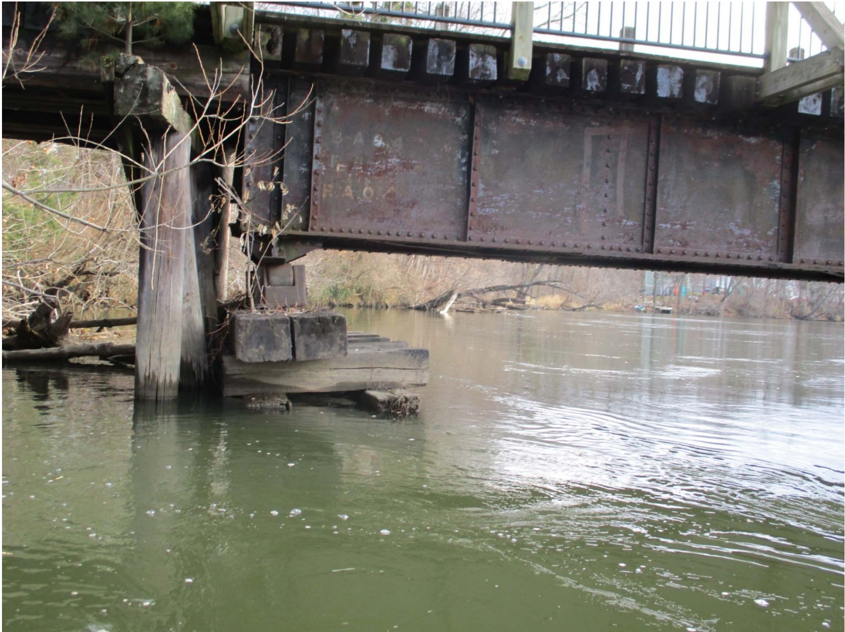
Pier 9S cribbing has settled and rotated north
