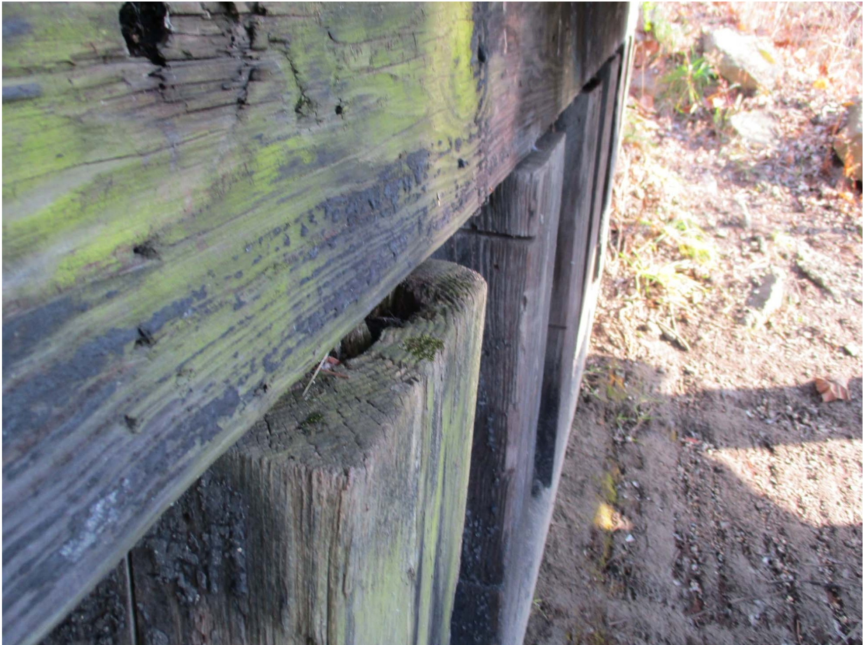
Internal rot to vertical supports at north abutment
