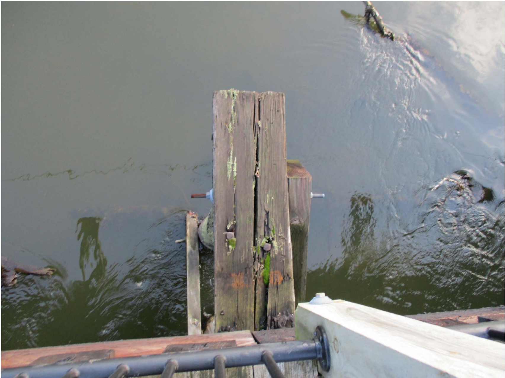
Pier 3S east end split, depressed section at beam, internal rot likely
