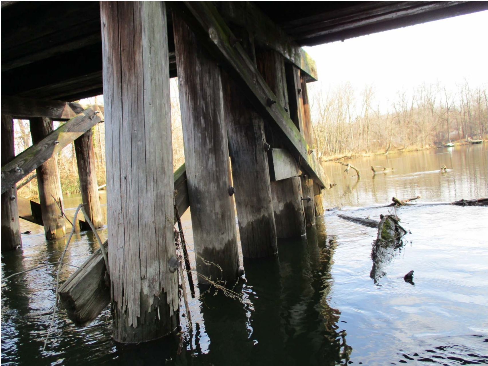
Pier 2S surface rot to pile 1W
