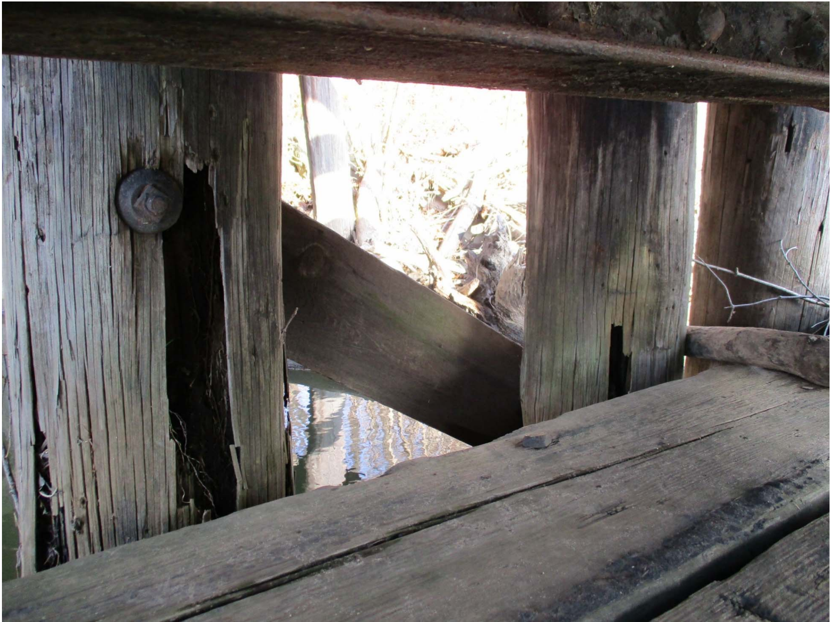
Pier 9S interior piles completely rotted through
