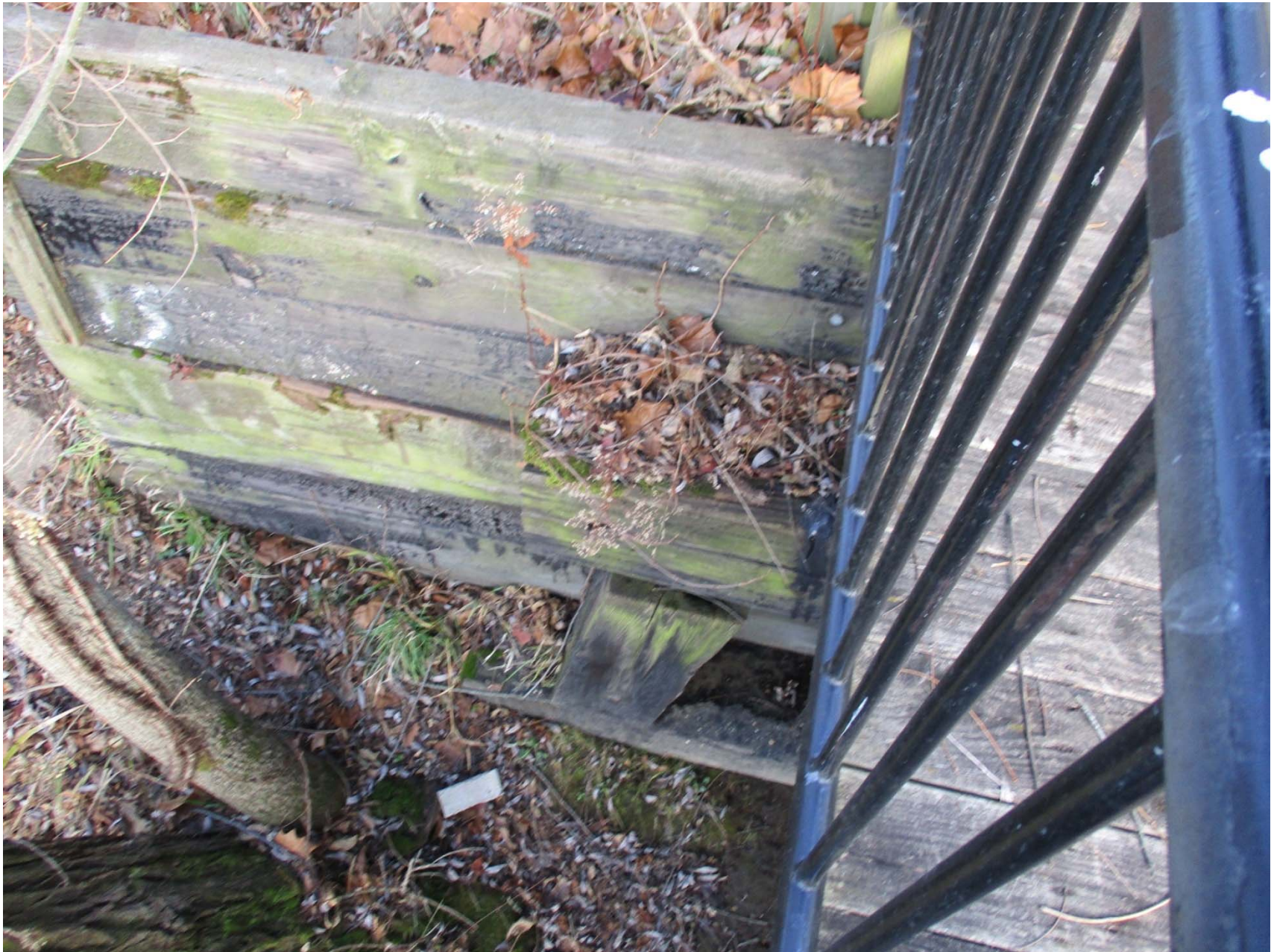
North abutment west end vegetation growth on cap
