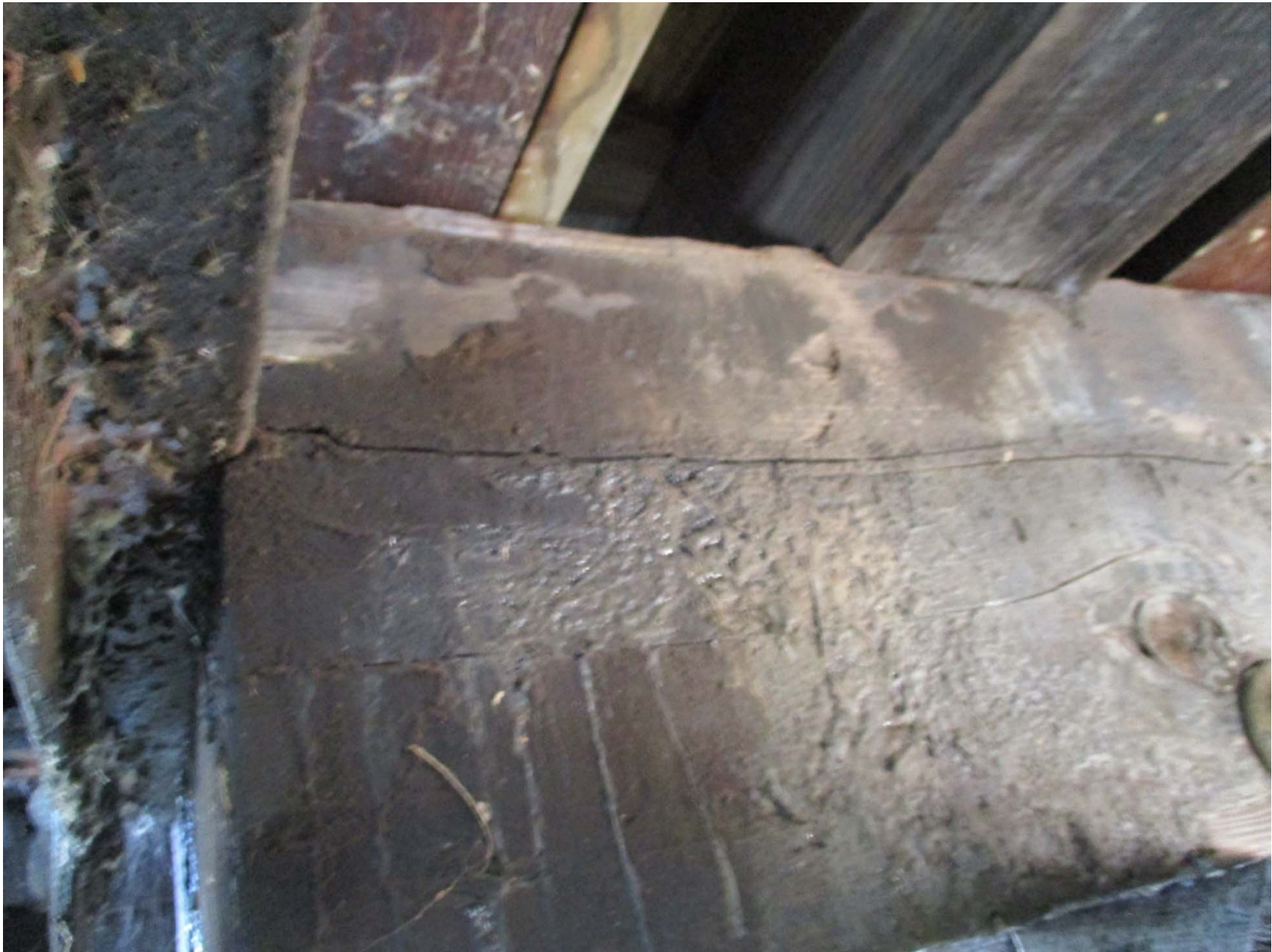
West beams splitting where bearing against the steel cross brace angle
