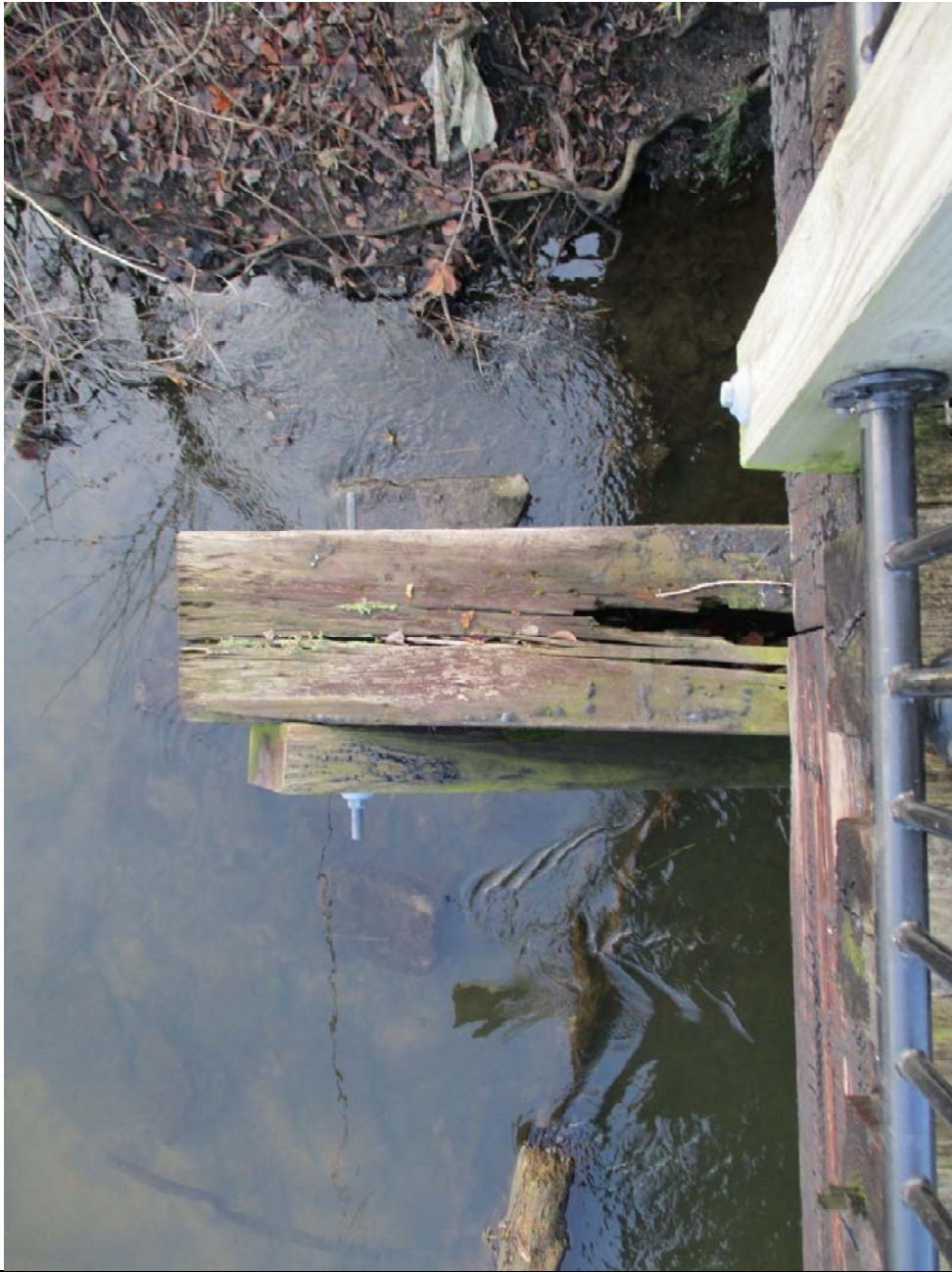
Pier 1S east end rotted
