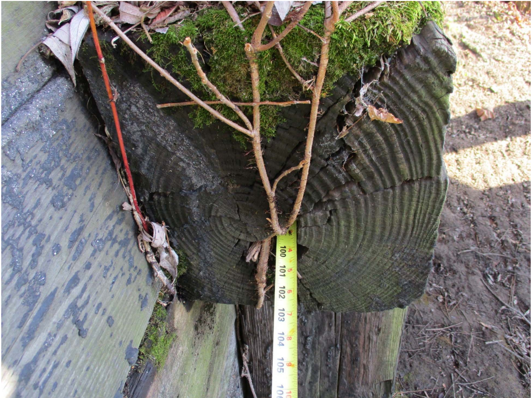
North abutment cap internal rot extends at least 100 inches from west end
