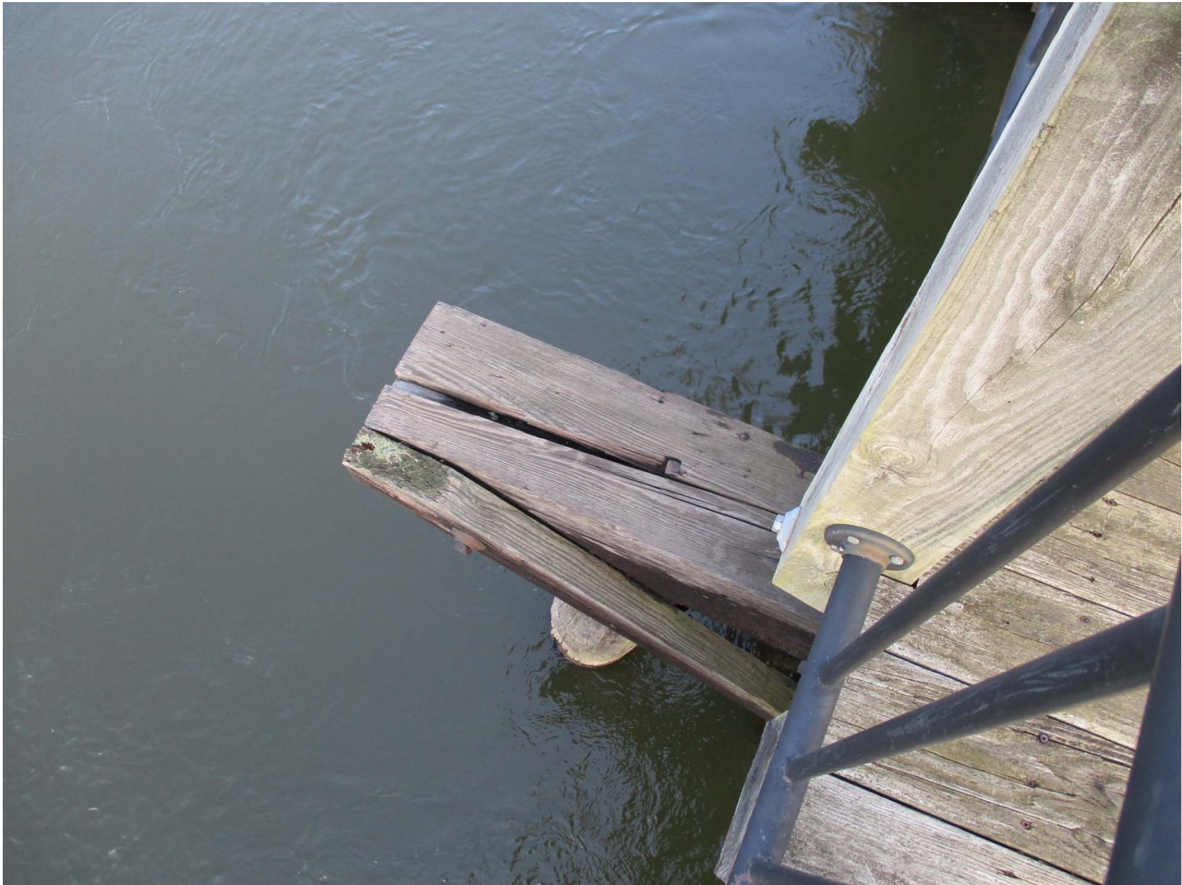
Pier 6S west end split with internal rot likely
