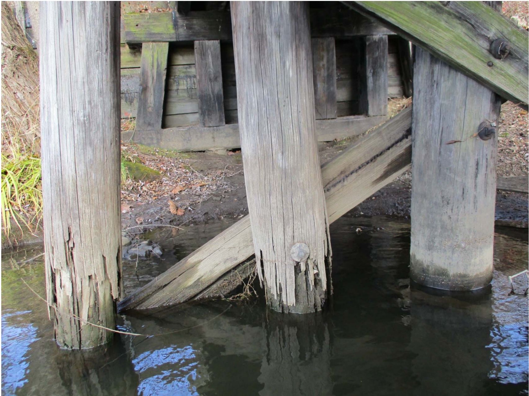
Pier 10S pile rot at water line
