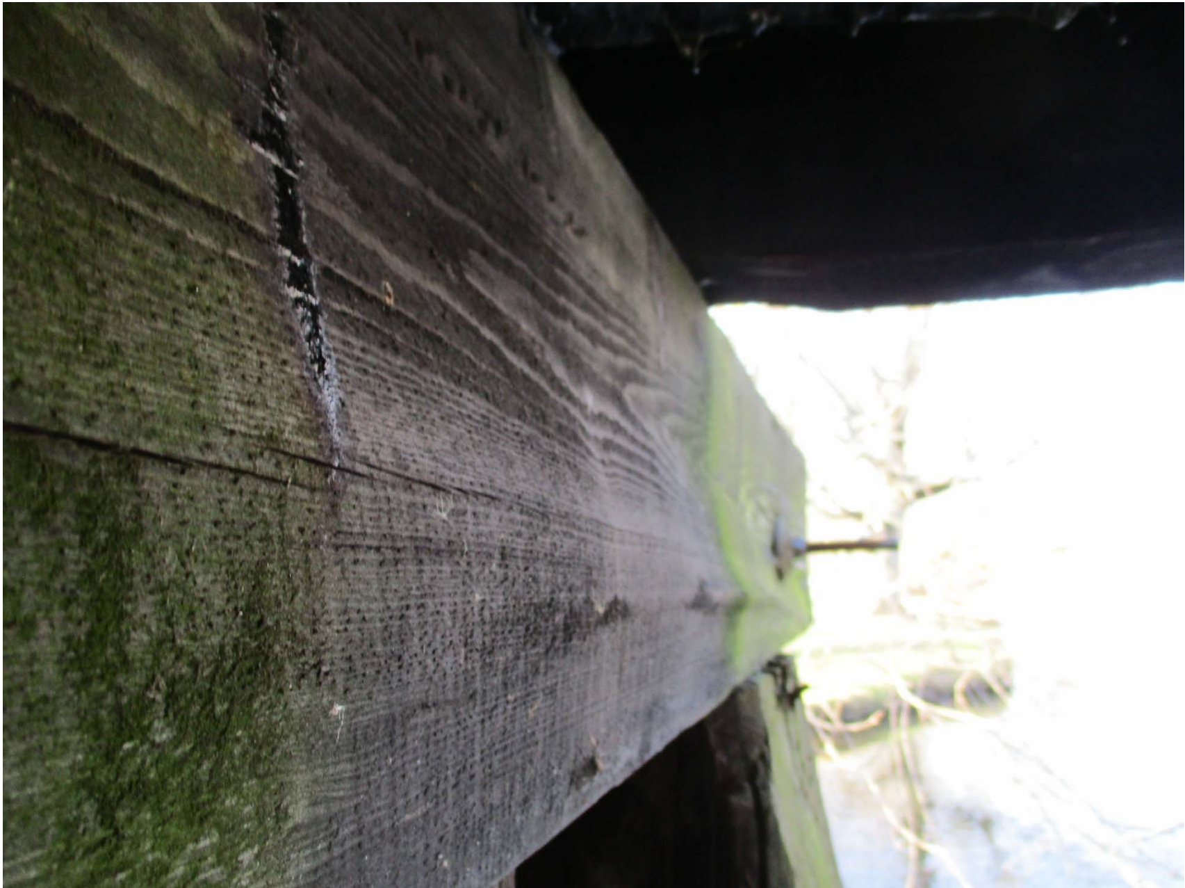
Pier 1S west end crushing/buckling
