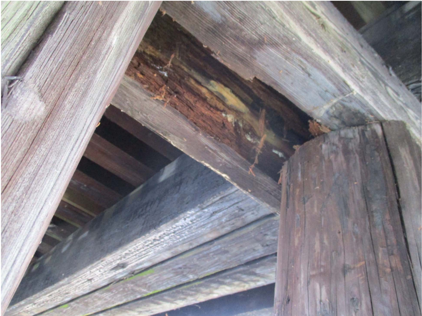
Pier 3S cap internal rot with fungus growth
