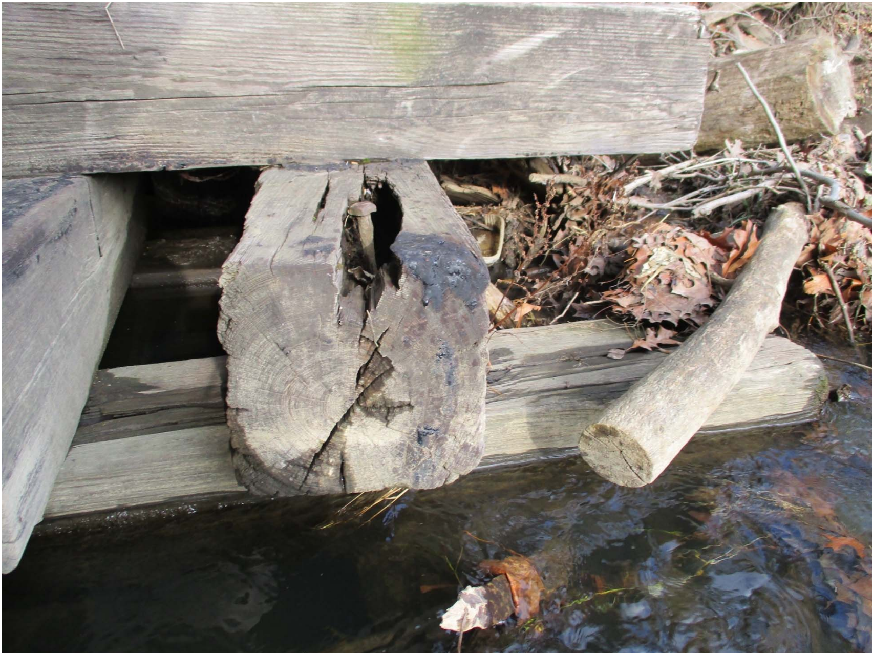
Pier 9S north end cribbing rotted
