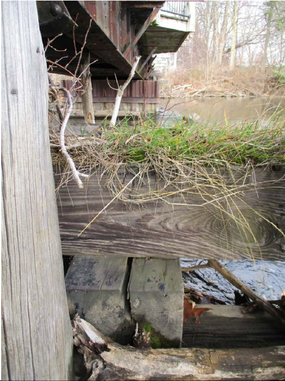
Steel beam cribbing split, vegetation growing out of upper timbers at pier 7S
