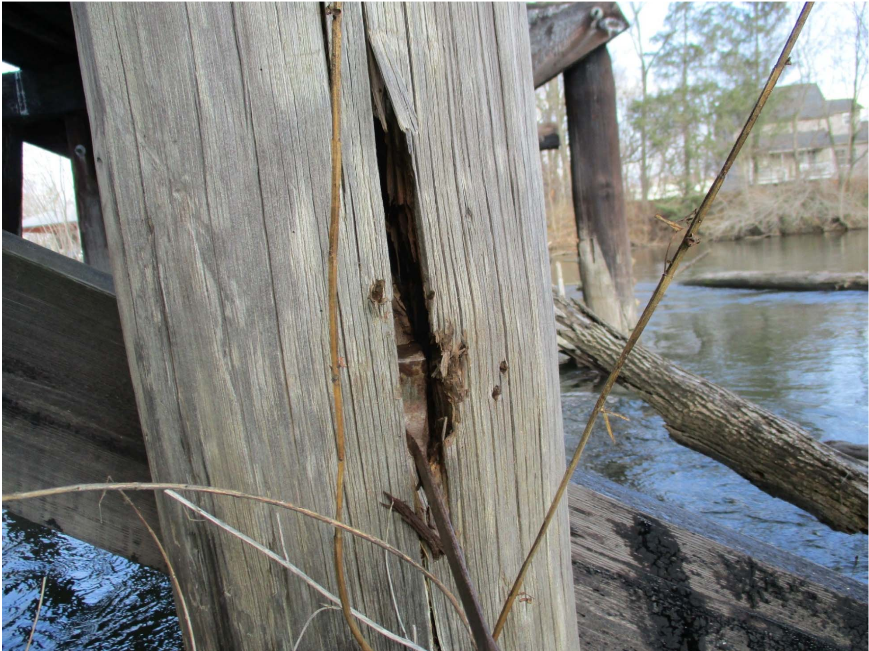
Pier 4S pile 3W internal rot
