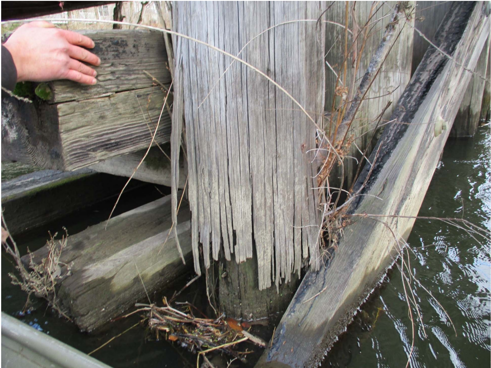
Pier 7S pile rot at water line
