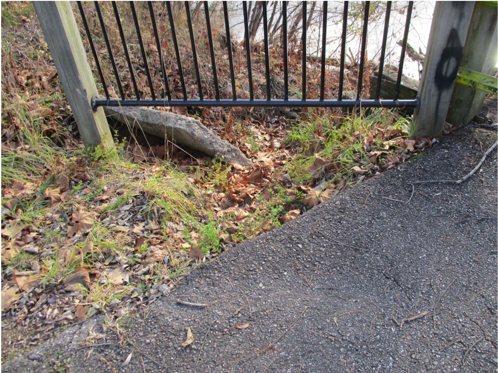
Erosion beginning to undermining approach path along east side
