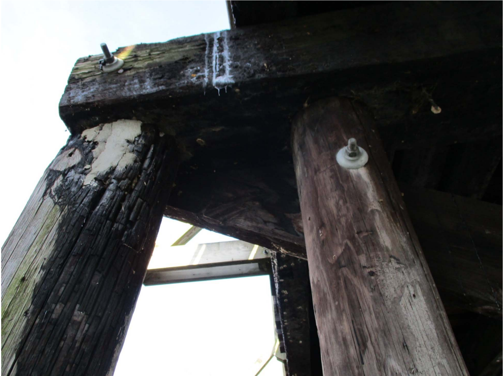
Pier 5S pile 1W has fire damage
