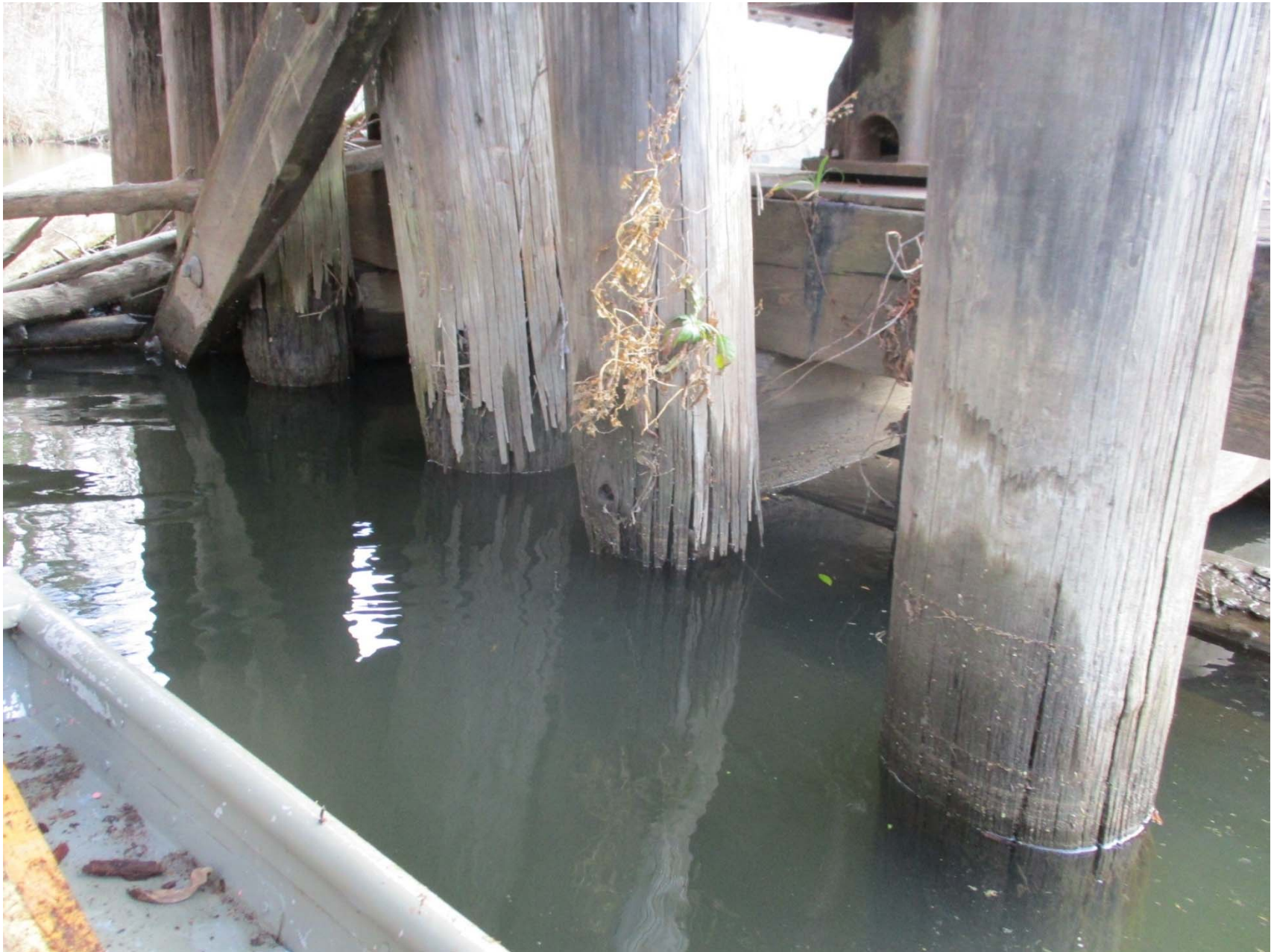
Pier 9S pile rot at water line
