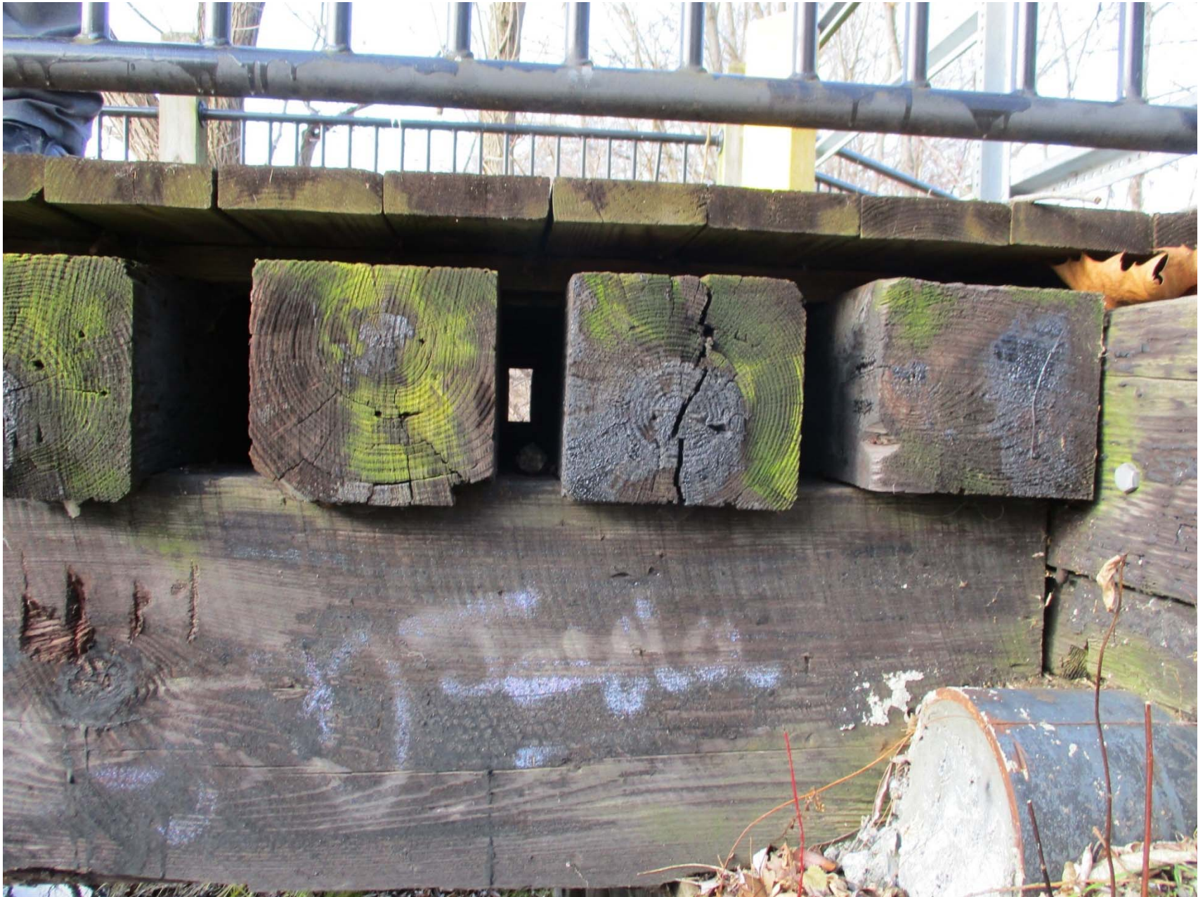
Scattered end split ties with some rot
