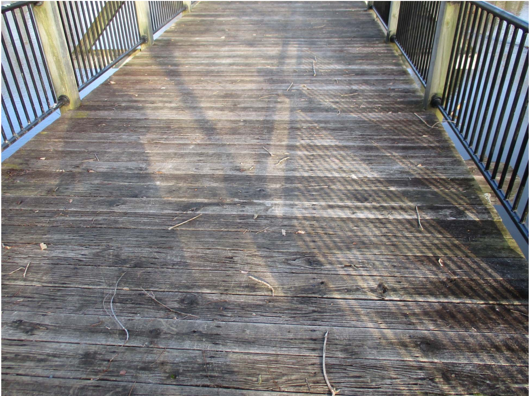
Decking is weathered and checked. Fasteners are rusting.
