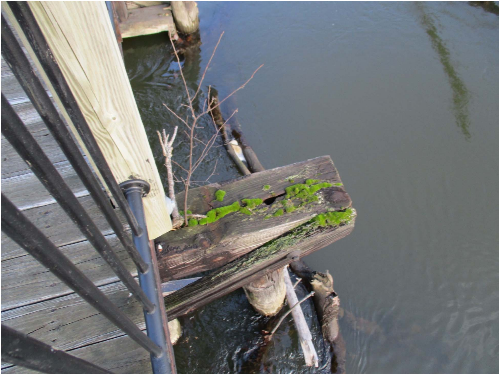
Pier 4S east end with internal rot with tree growth
