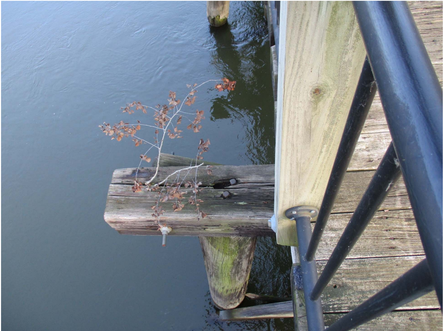
Pier 3S west end rotted with tree sapling growing
