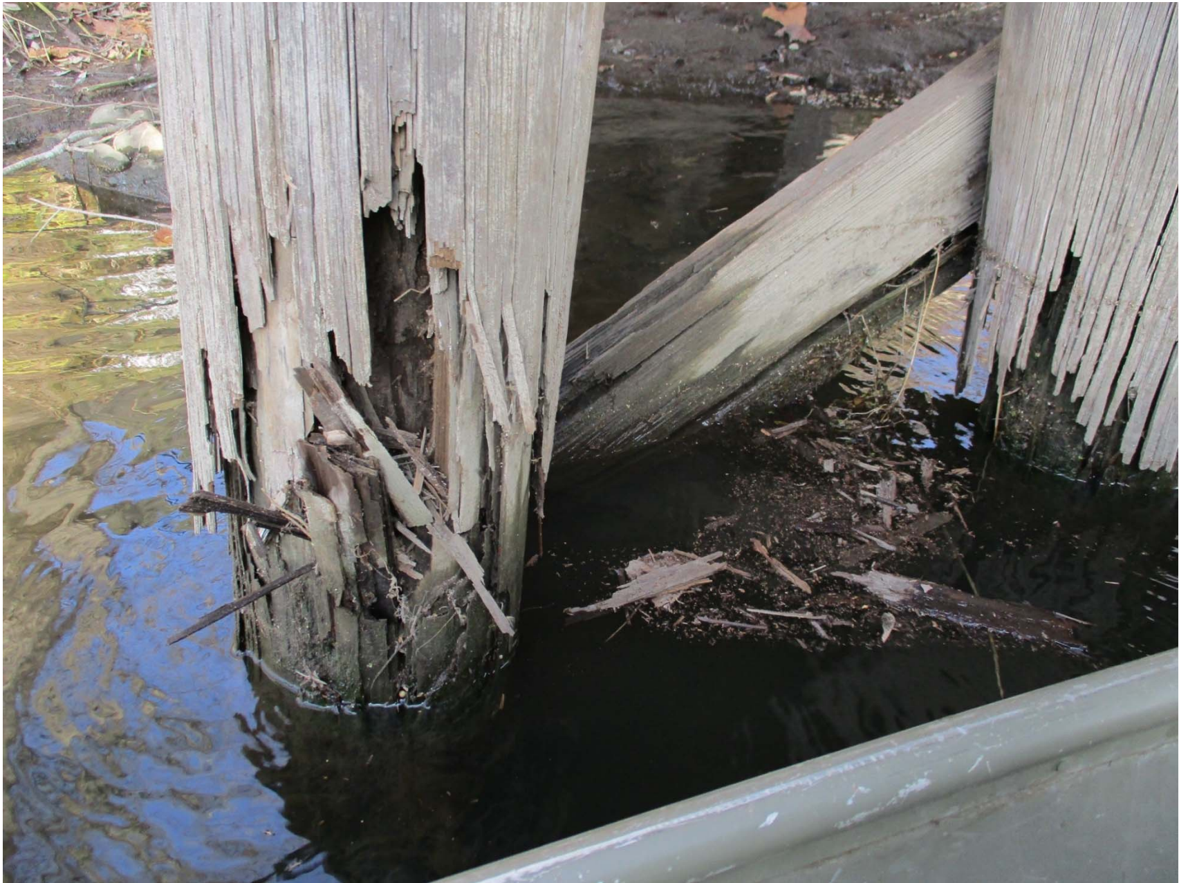
Pier 10S Pile 1W, 60-70% loss
