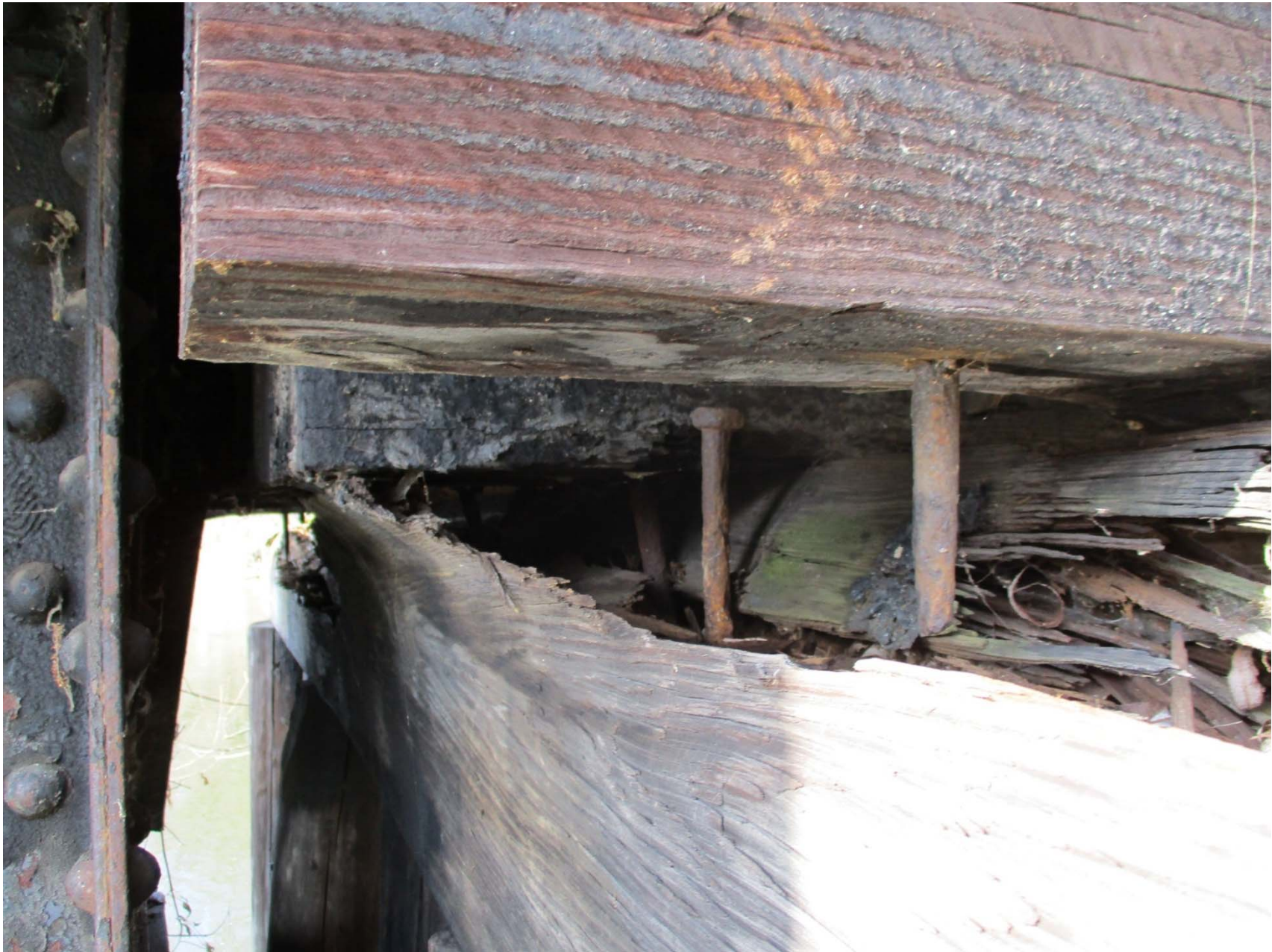
Pier 9S east end cap rot
