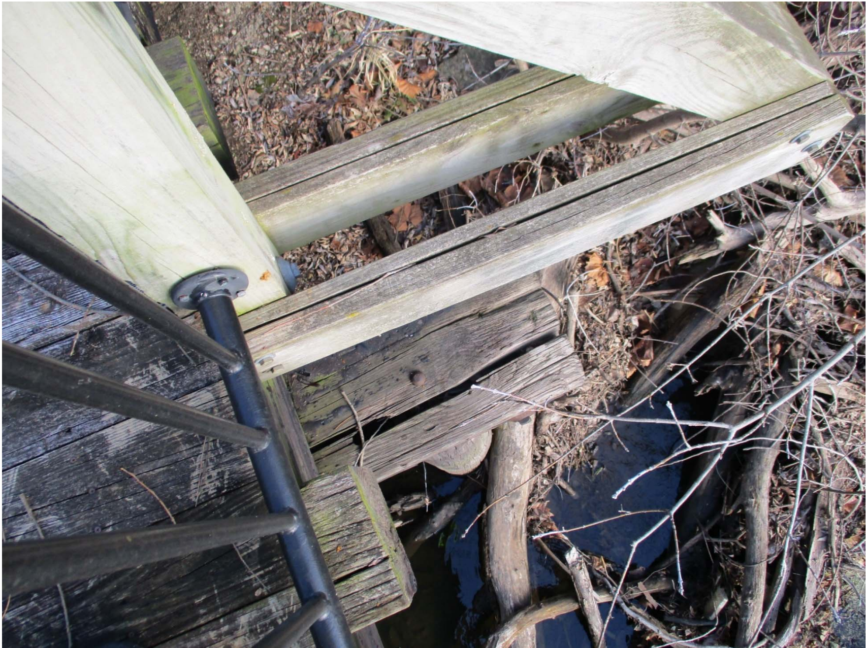
Pier 10S east end split with internal rot
