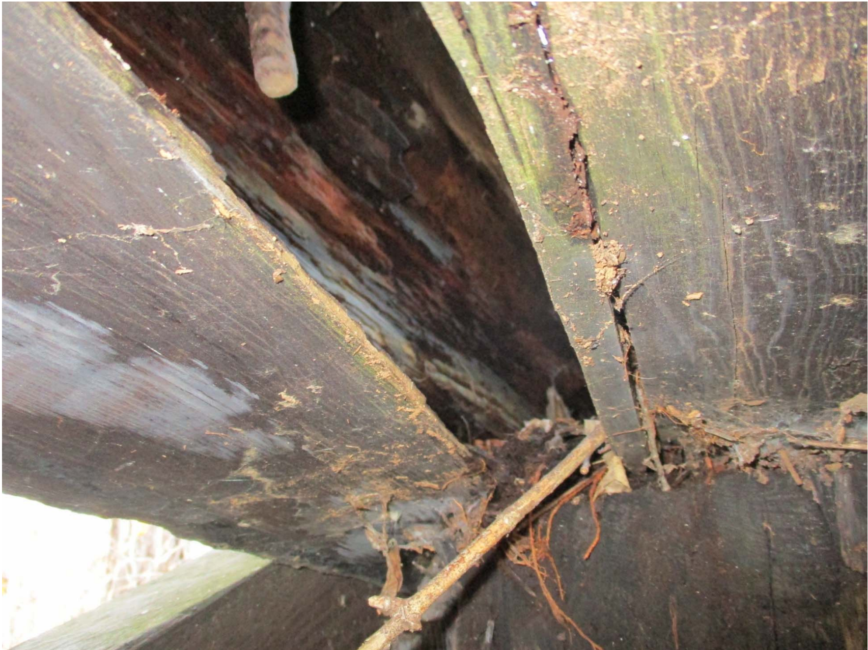
Pier 1S east half rotted
