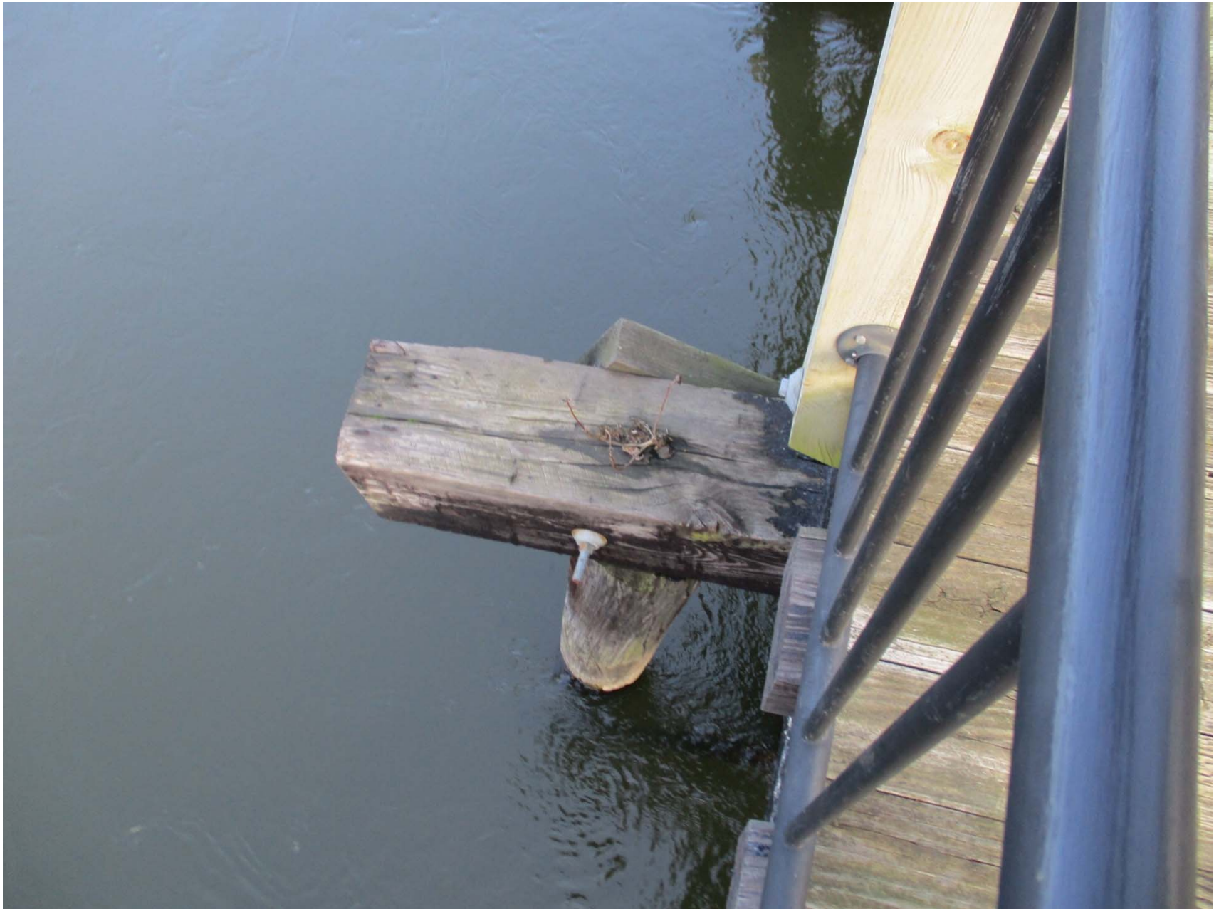
Pier 4S split with vegetation growing in bolt hole
