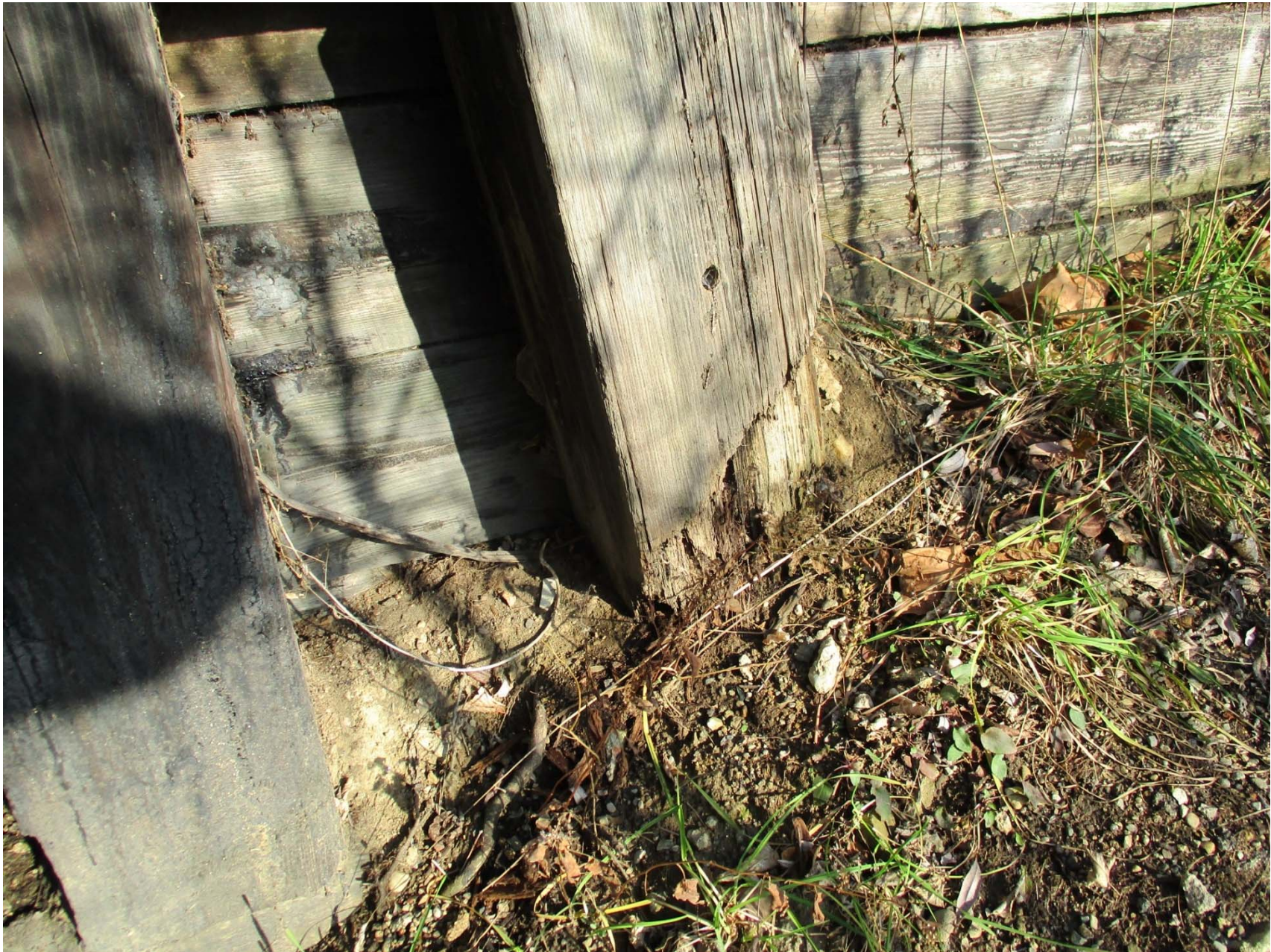
North abutment east pile rot at ground line
