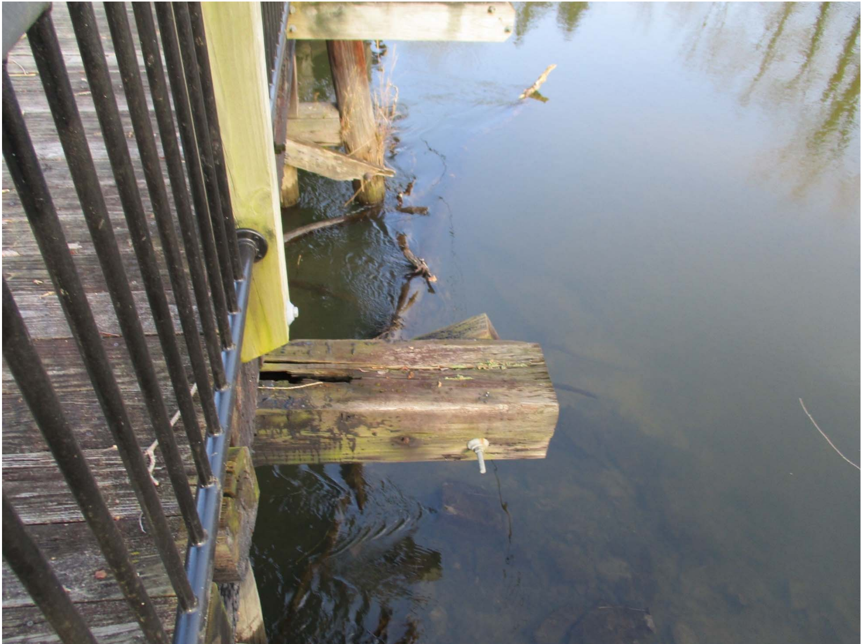
Pier 3S east end rotted interior
