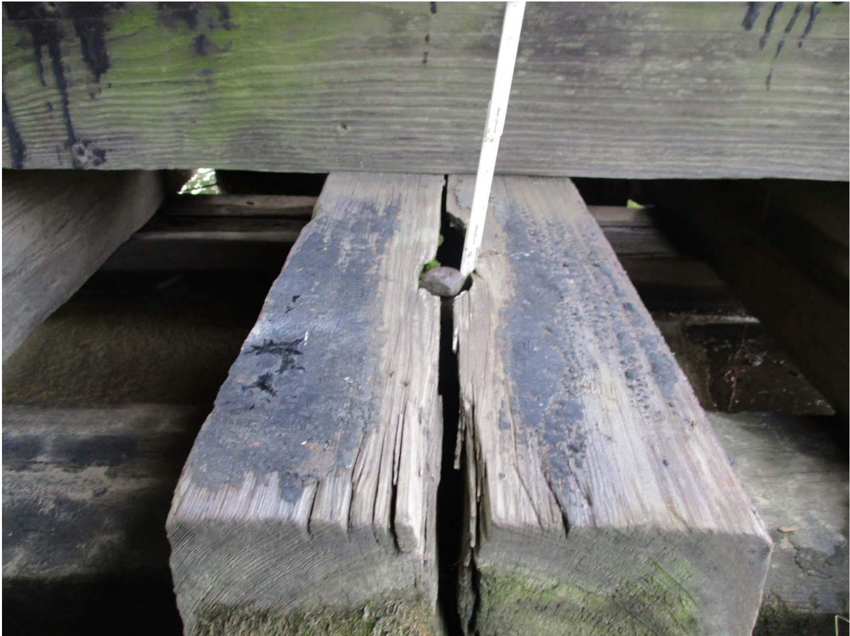
Pier 7S cribbing split with rot, west end
