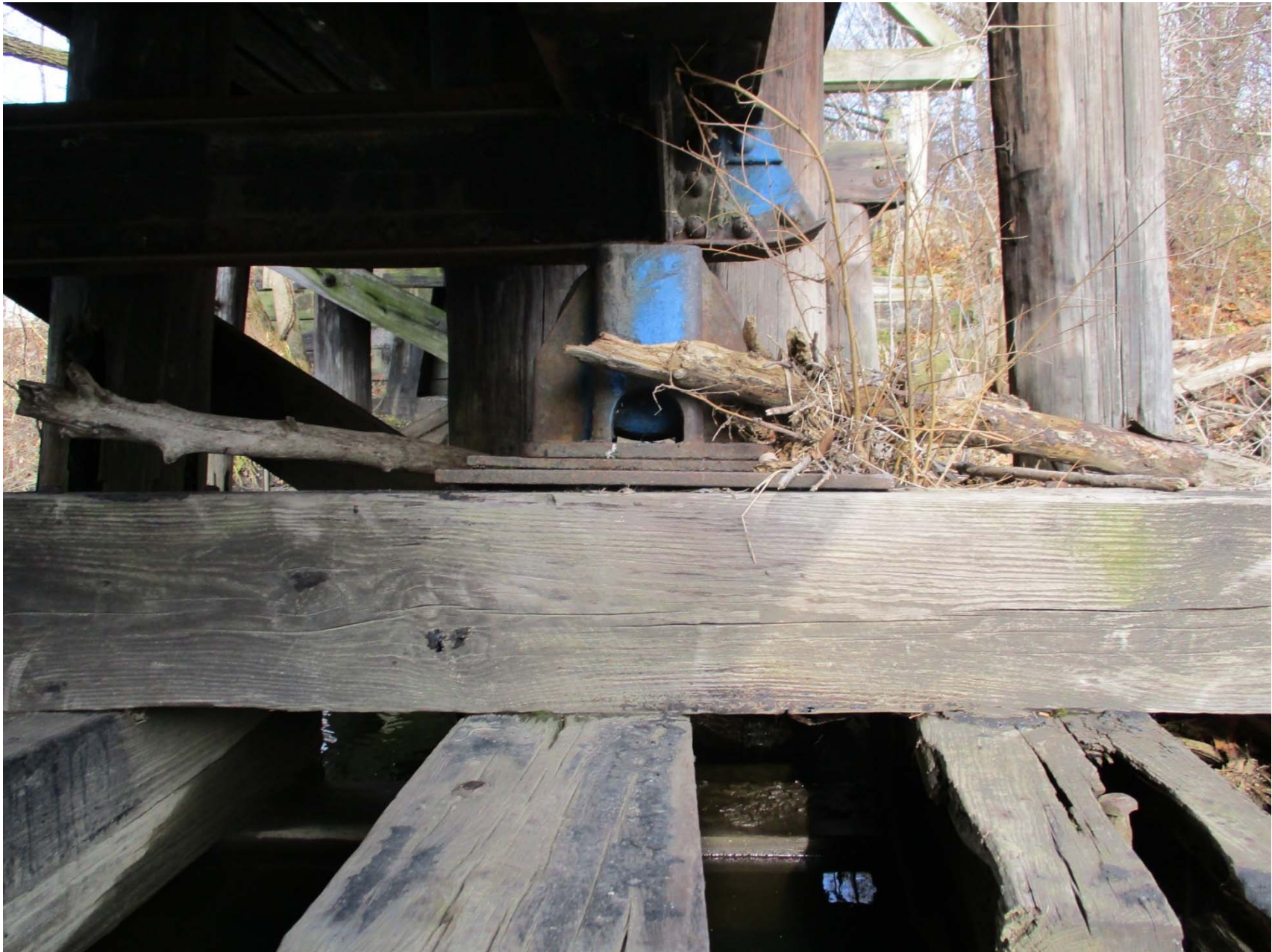
Gap between east bearing plates and cribbing at pier 9S
