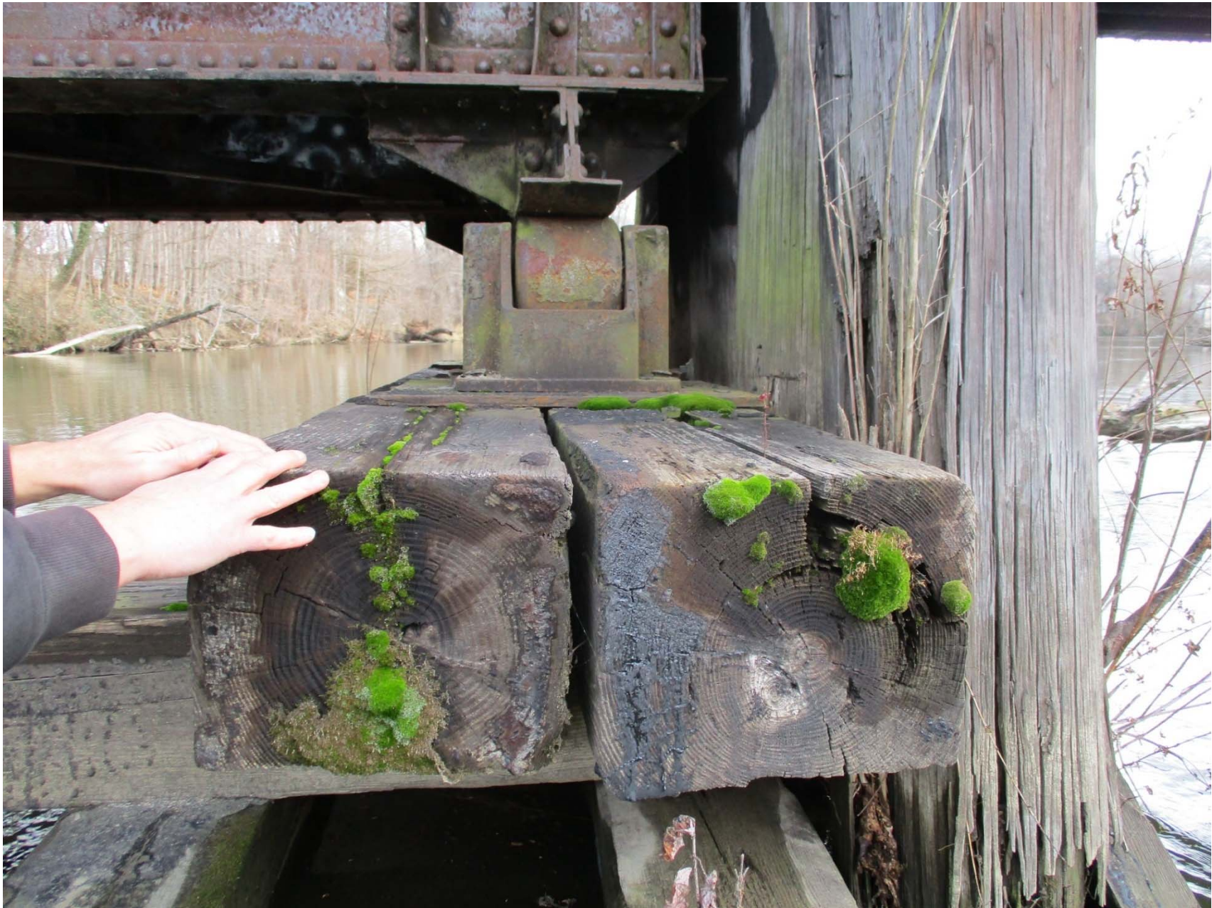
Pier 7S cribbing split with rot
