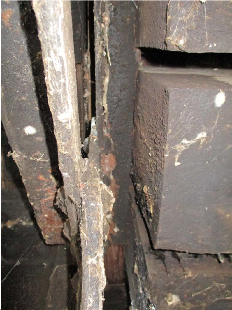
Span 10S is being held up by west beams pressing against a steel cross brace angle
