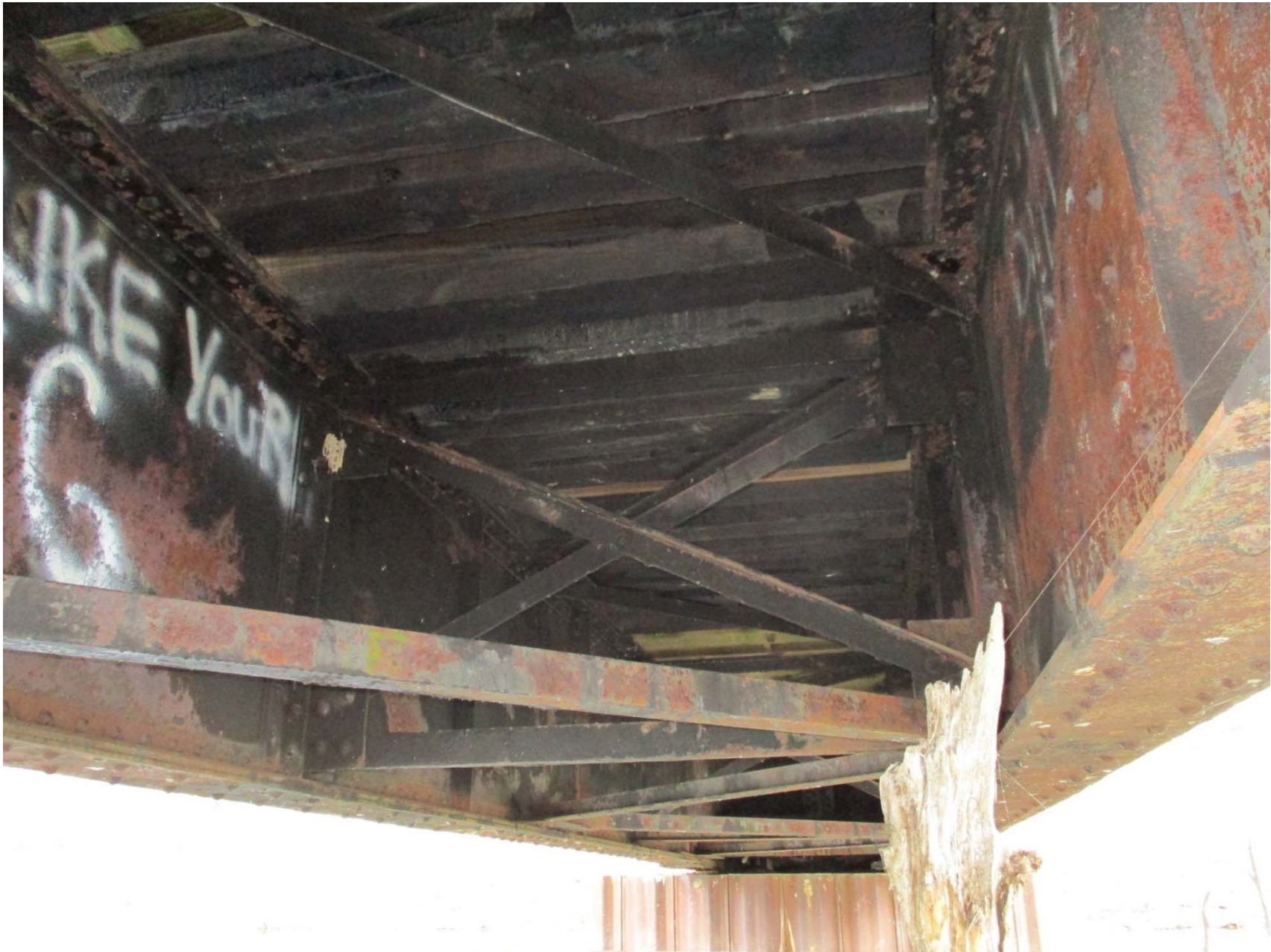
Light rust to steel beams and bracing
