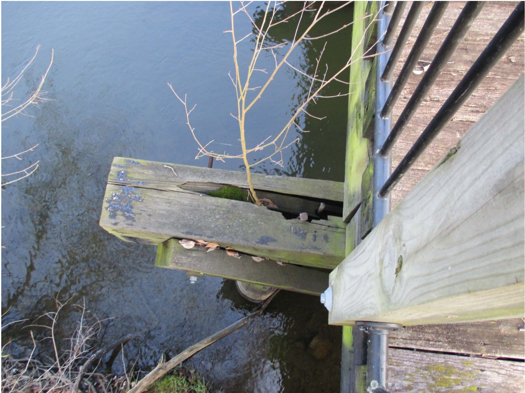
Pier 1S west end interior rotted with only an exterior shell left in place, tree growing in rotted interior
