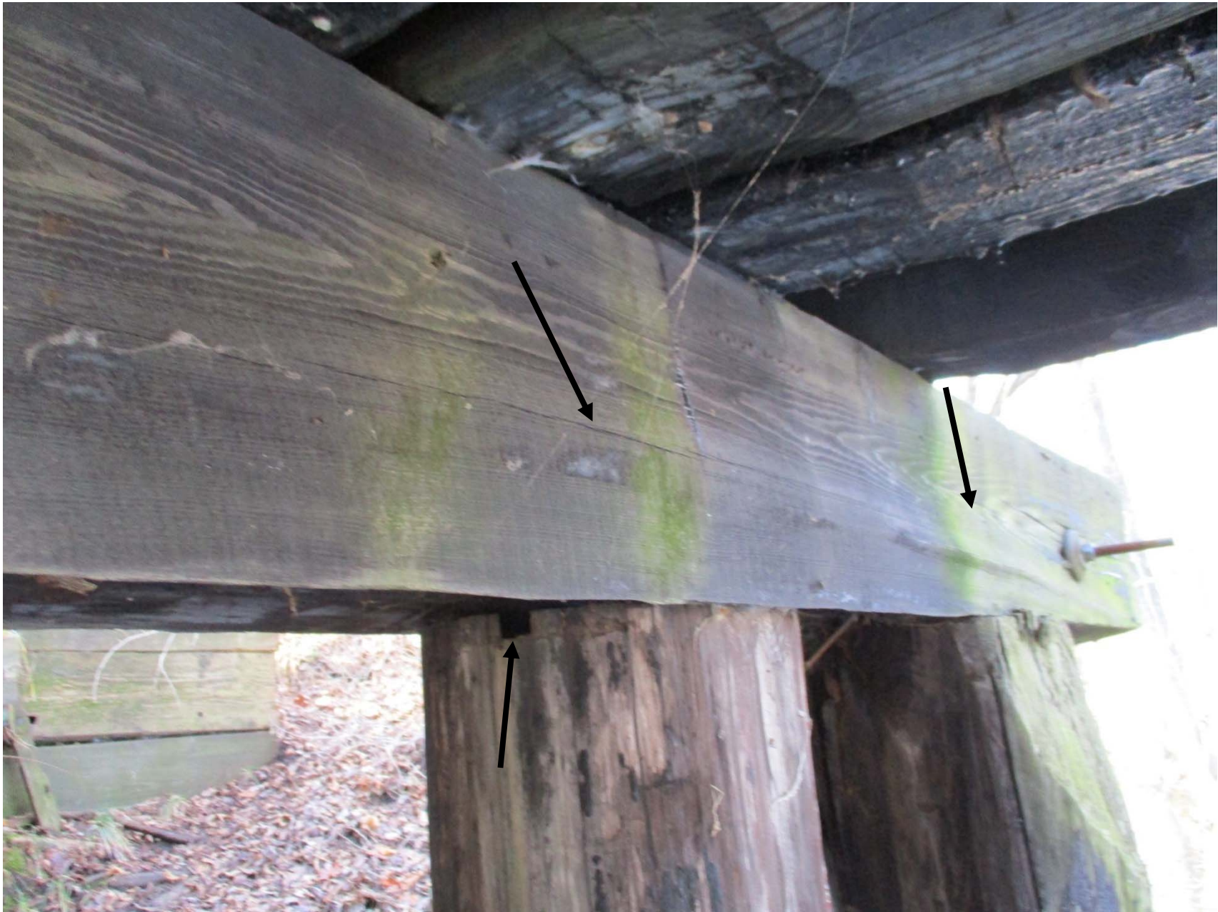
Pier 1S west end of remaining cap is crushing, rot inside top of piles
