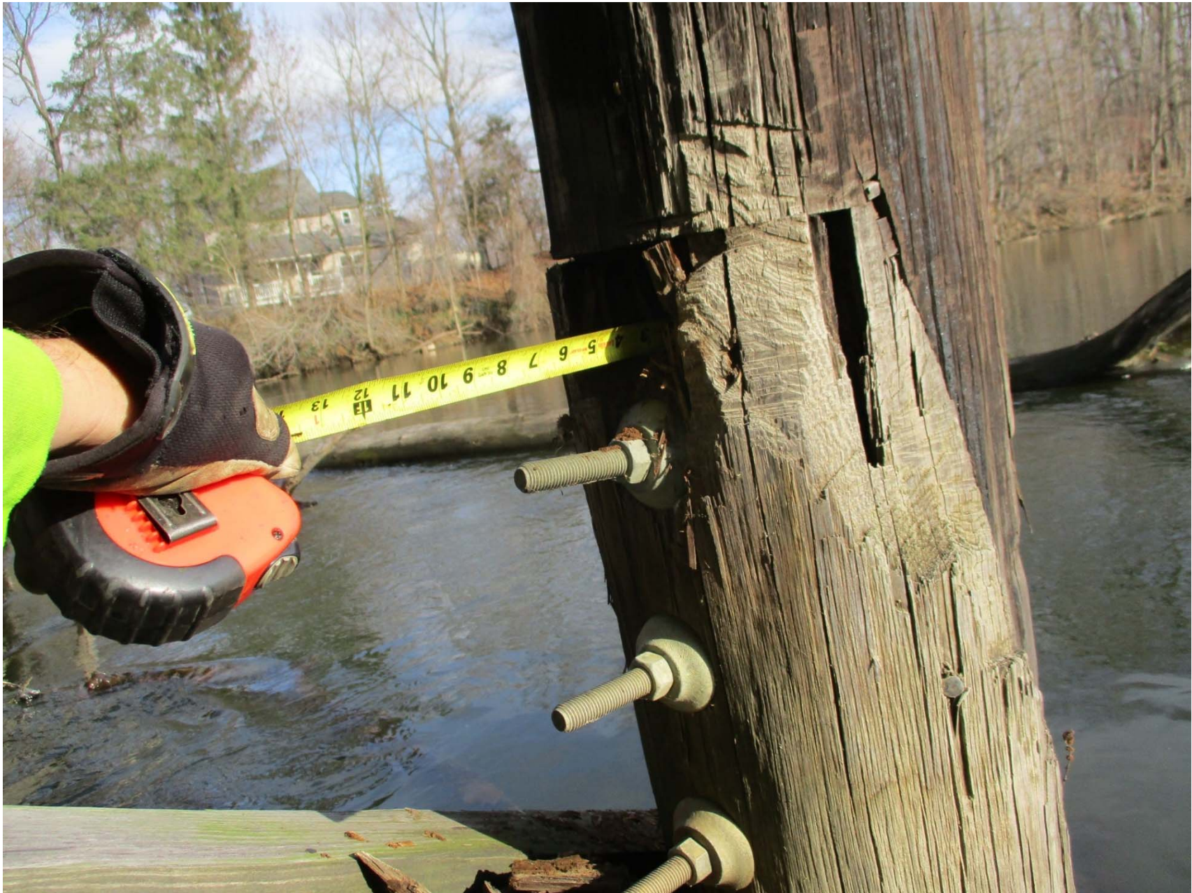
Pier 5S pile 1E lower west half rotted
